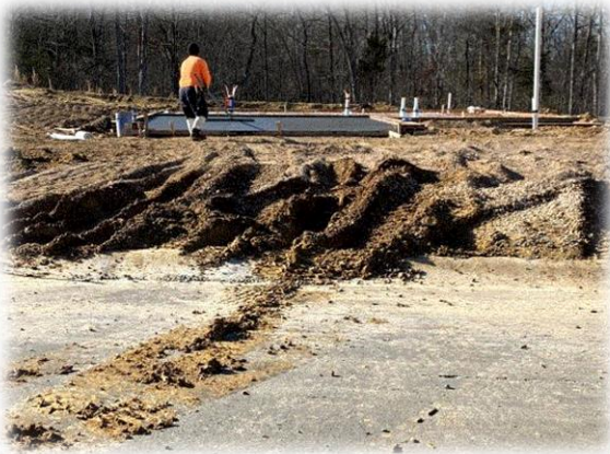
Figure 8 - Poor Construction Entrance
