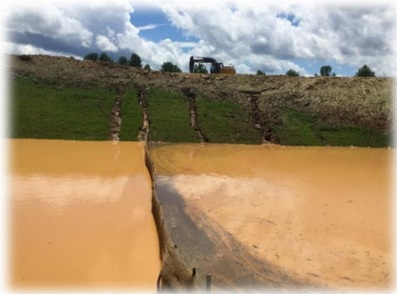
Figure 11 - Rill Erosion on Sediment Basin Slope
