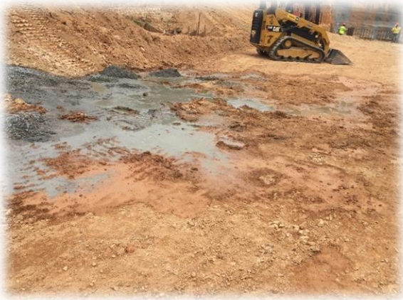
Figure 6 - Unmanaged Concrete Washout
