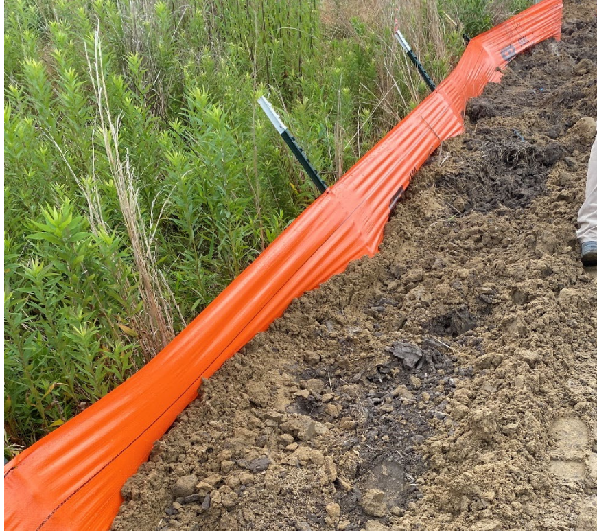
Silt fence being pushed over
