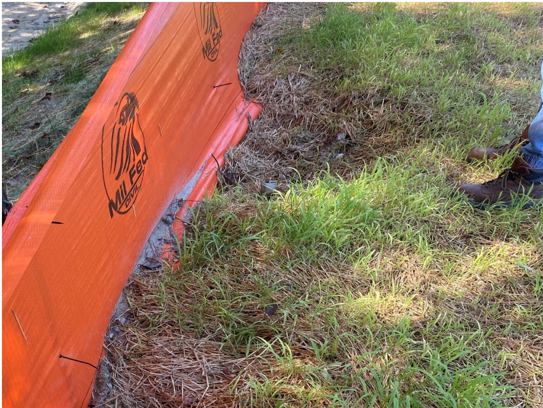
Silt fence undermined
