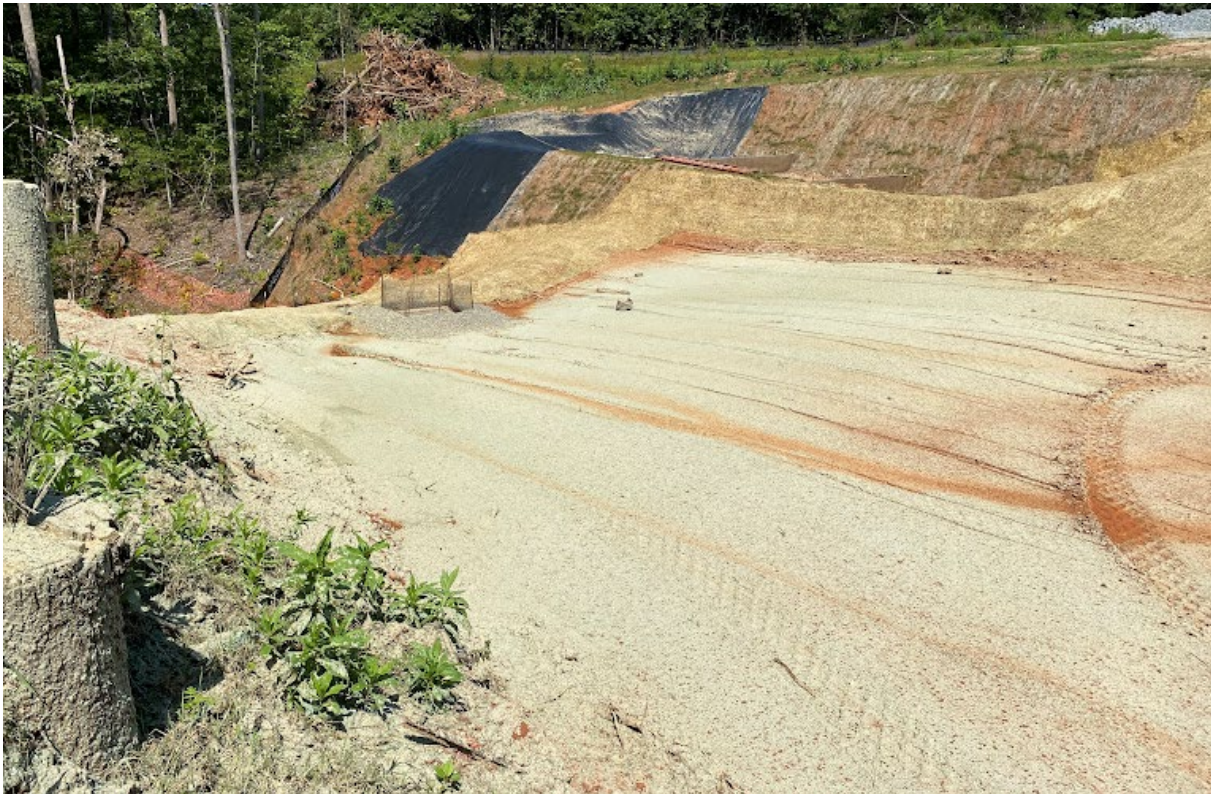
Basin and drop inlet protection measure
