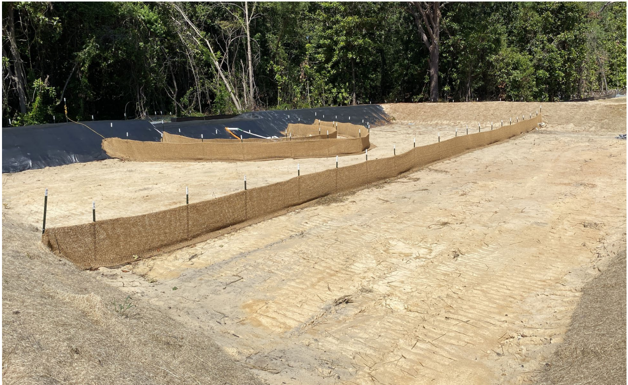
Recently installed basin
