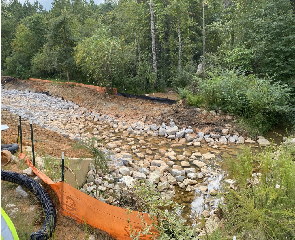
Channel adjacent previously noted sediment loss
