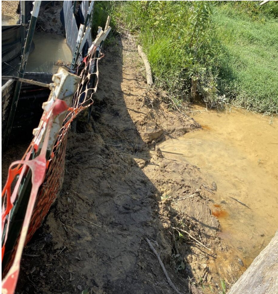
Sediment noted beyond silt fence adjacent to channel change
