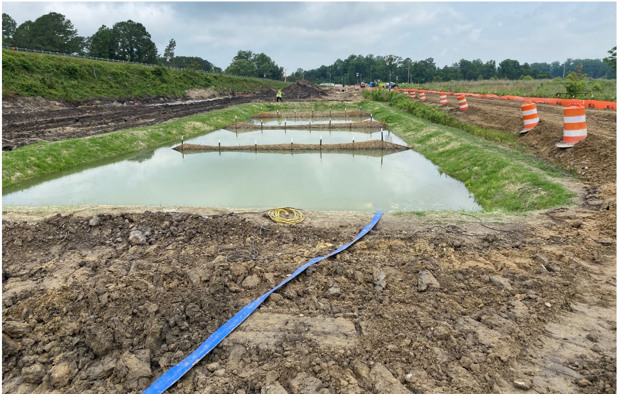
Skimmer device not installed, and diversion ditch not yet tied into basin
