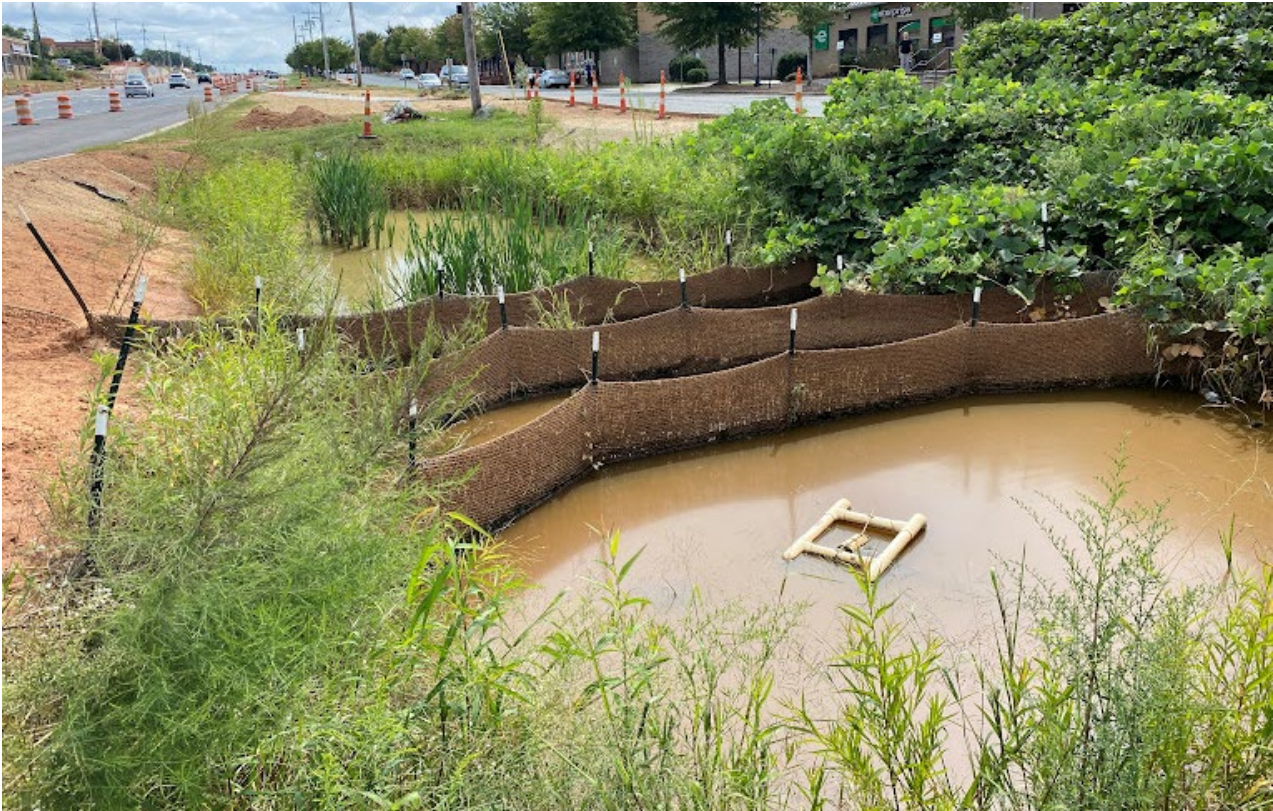
Baffles not properly spaced
