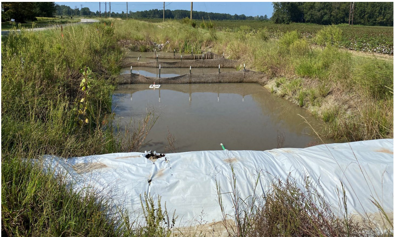
Skimmer device detached and spillway liner damaged
