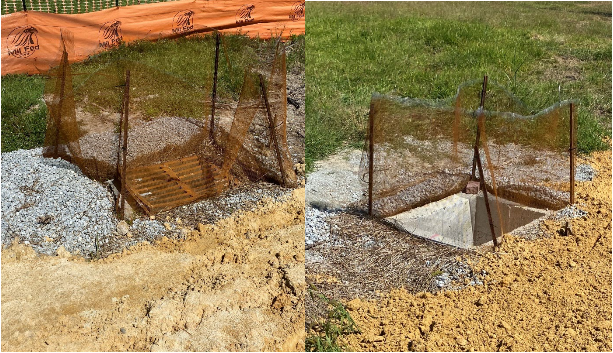
Drop inlet protection measures needing maintenance
