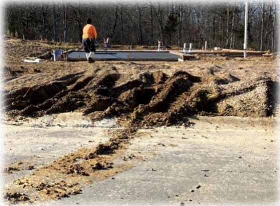
Figure 8 – Poor Construction Entrance
