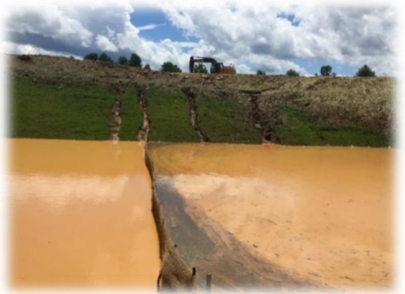
Figure 11 - Rill Erosion on Sediment Basin Slope
