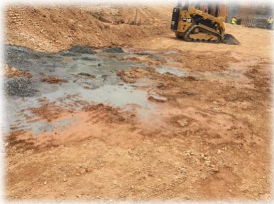
Figure 6 - Unmanaged Concrete Washout
