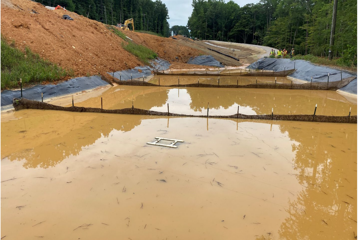
Slopes adjacent to skimmer basin needing stabilization.
