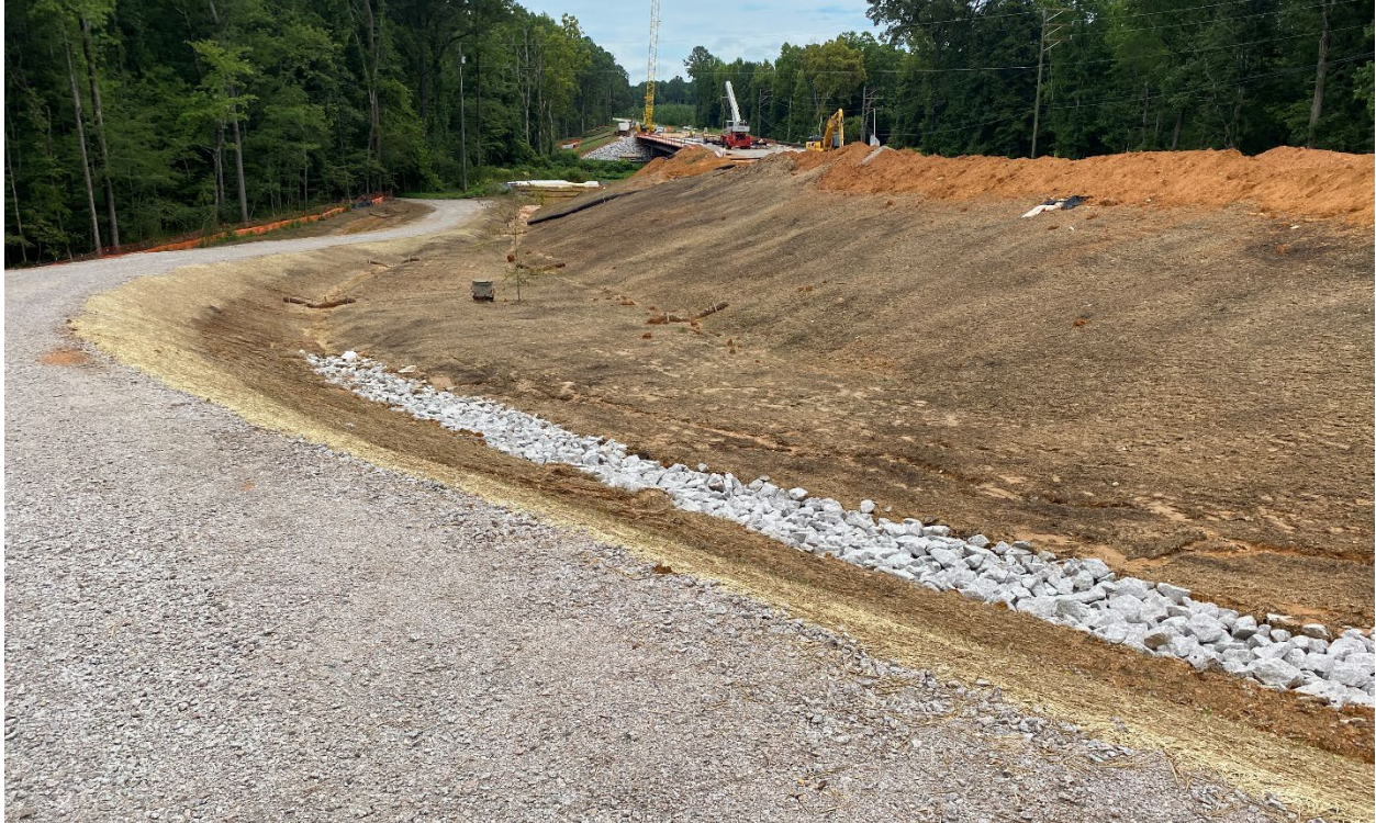
Areas seeded and mulched with straw; wattles recently replaced.
