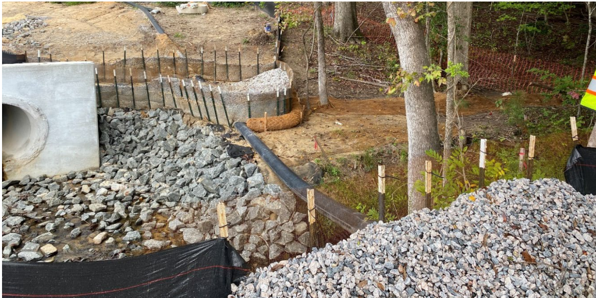
Additional measures installed and signs of previous loss cleanup.
