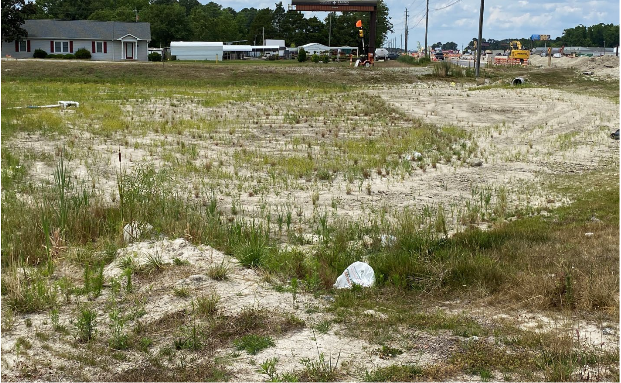
Permanent stormwater basin installed and being utilized as a skimmer basin during construction.
