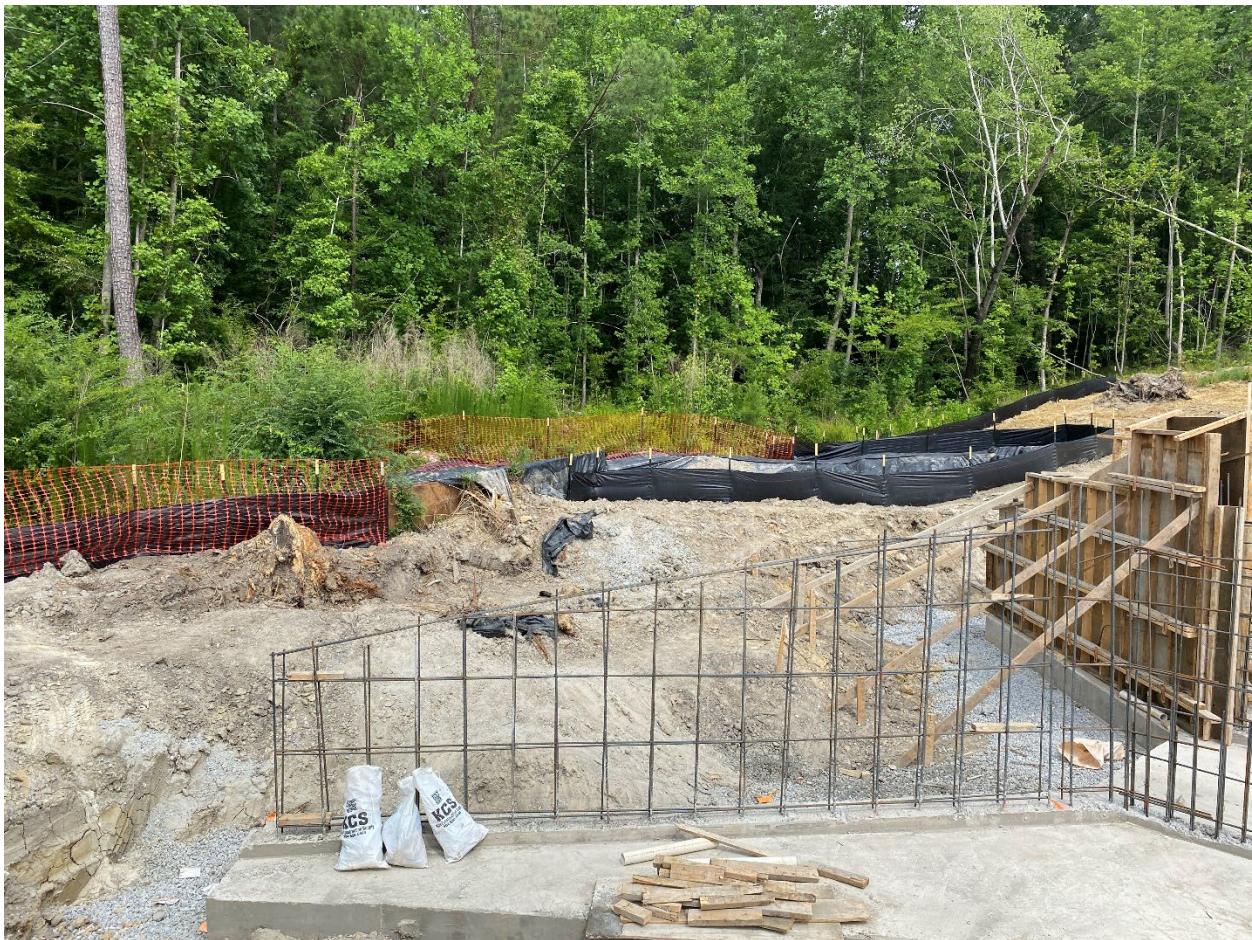
Headwalls of new culvert being installed and active temporary pipe outlet was protected.
