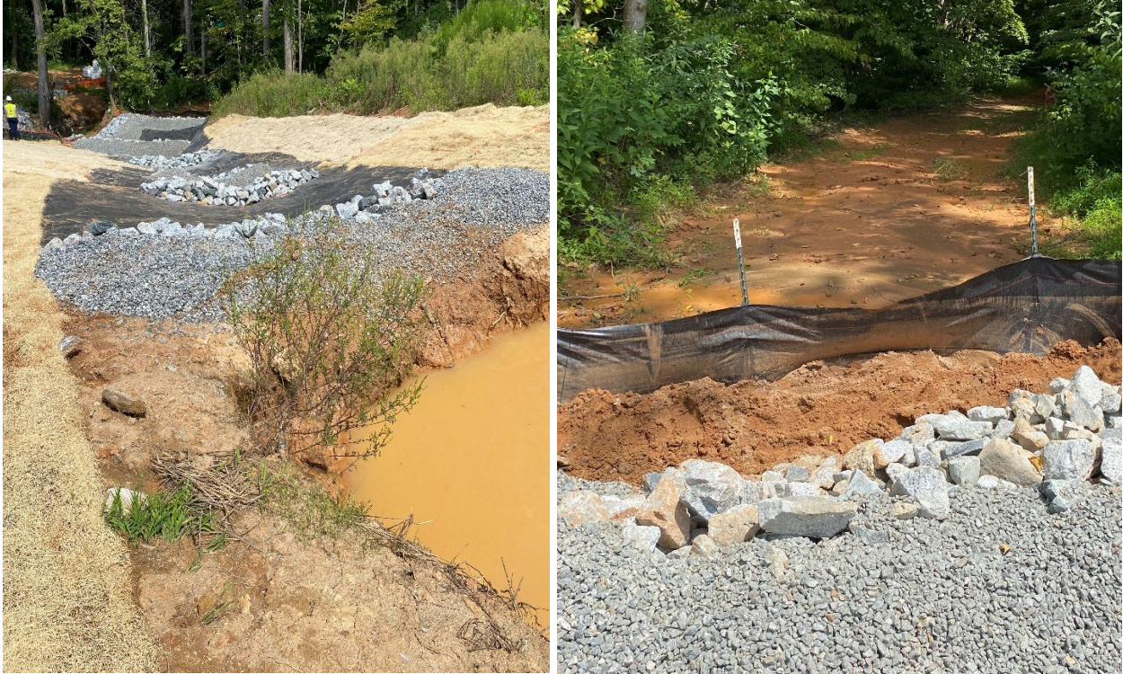
Repairs completed to area where sediment loss recently occurred, remaining sediment loss retrieval needed.
