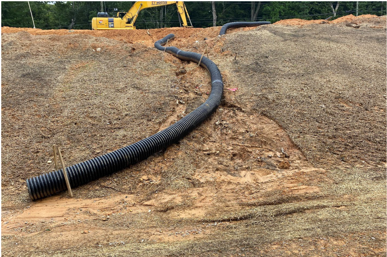
Slope drain recently added needs outlet protection measure and slope repairs.
