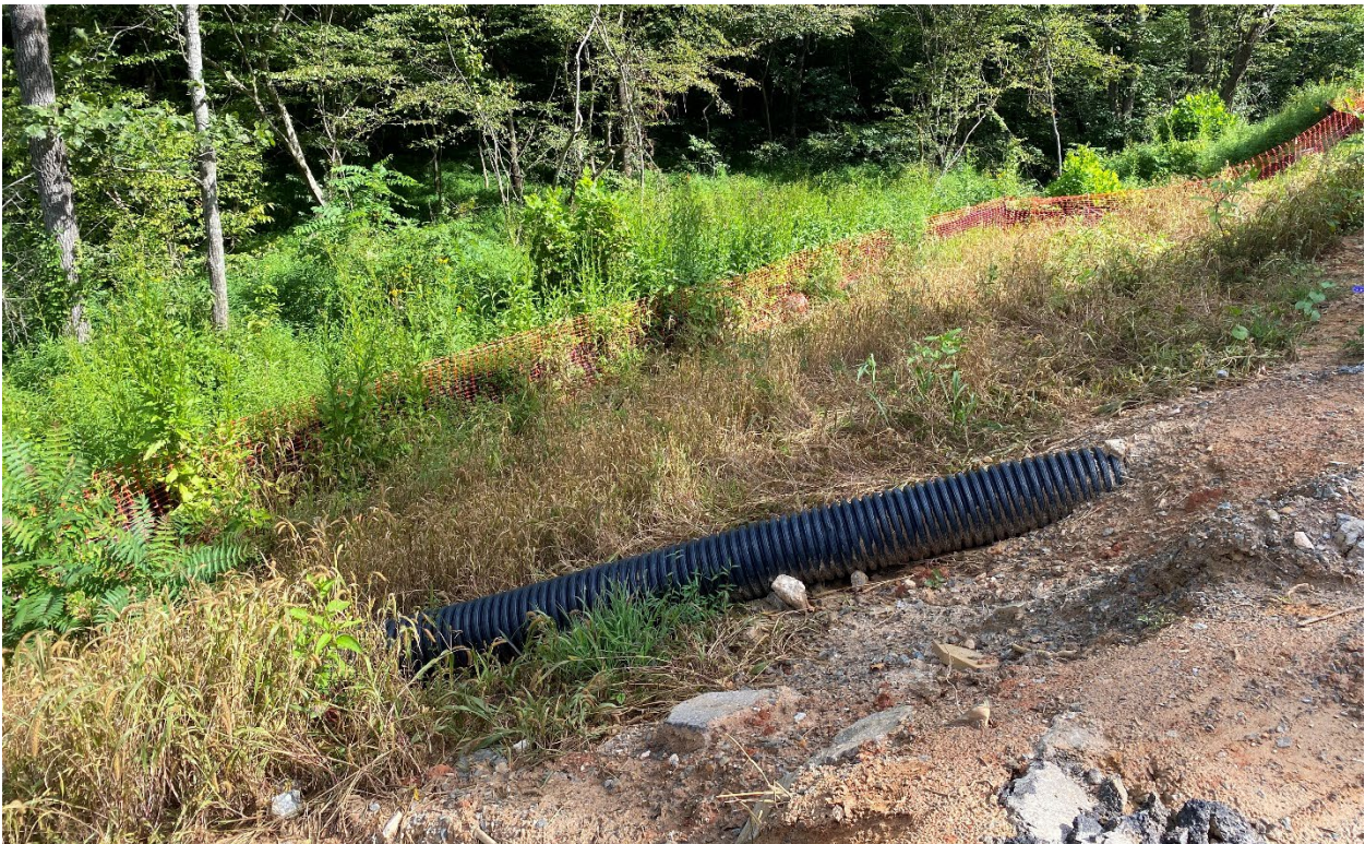
Vegetation starting to die out along stabilized slopes.
