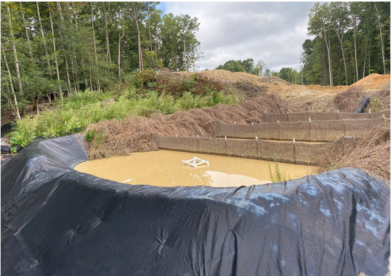
Skimmer basins maintained.
