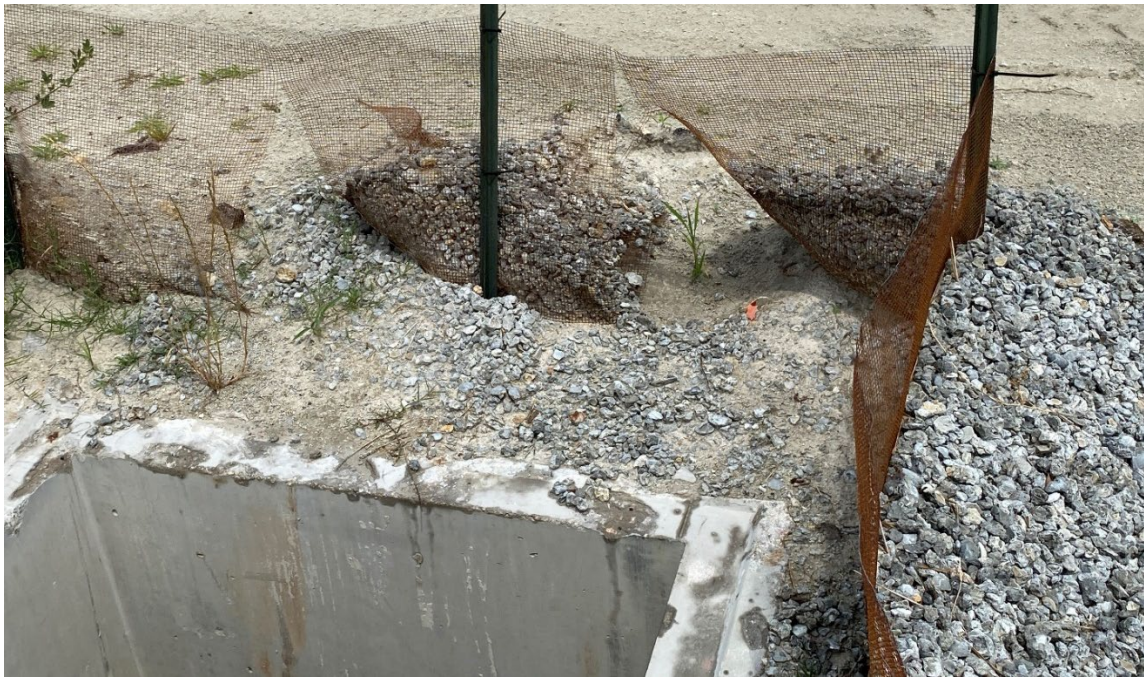
Drop inlet protection measures needing to be maintained.
