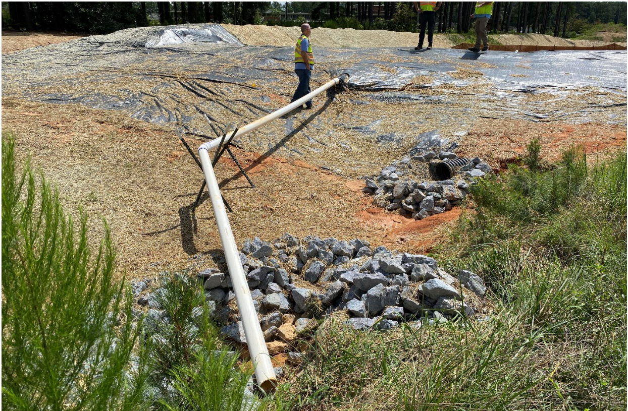
Recently repaired skimmer basin and extended skimmer device outlet.
