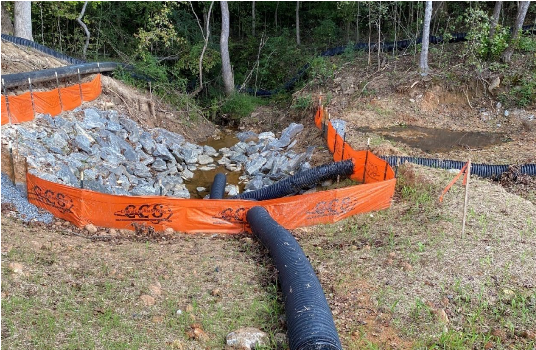
Slope drains extended beyond perimeter measures along stream bank.
