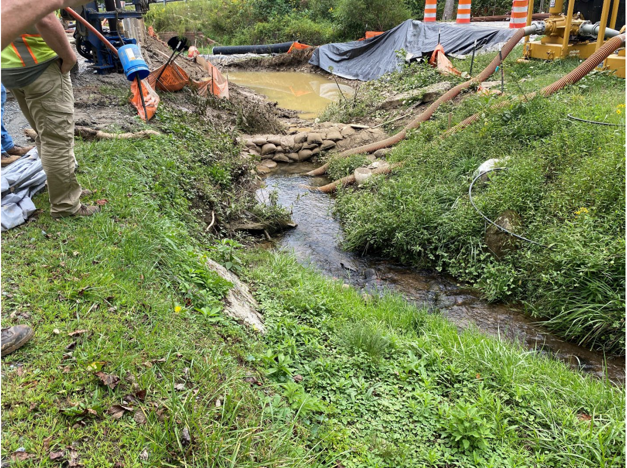
Recommended moving impervious dike and pump around operation at active culvert installation.
