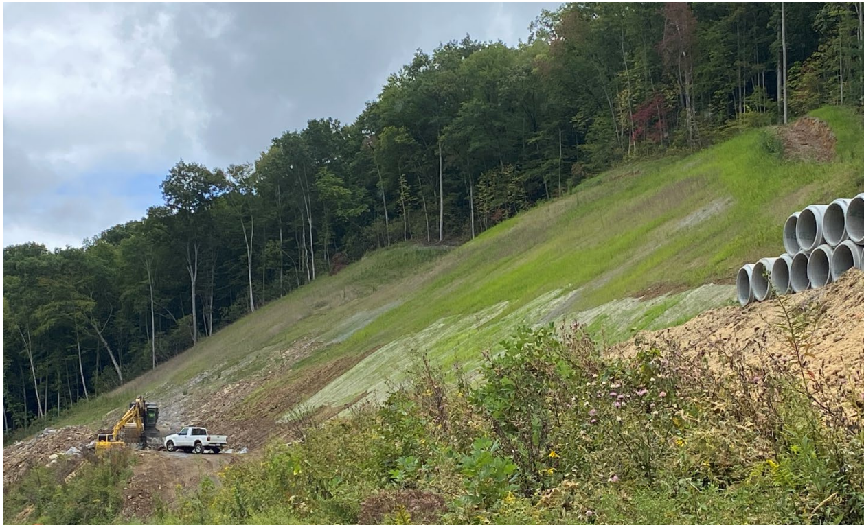
Cut slope being stabilized and clean water diversion along top of slope.
