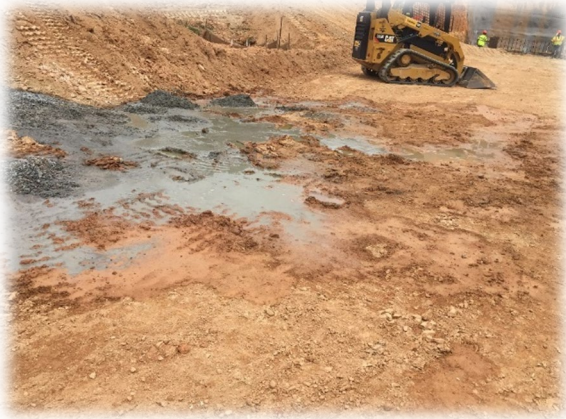
Figure 6 - Unmanaged Concrete Washout
