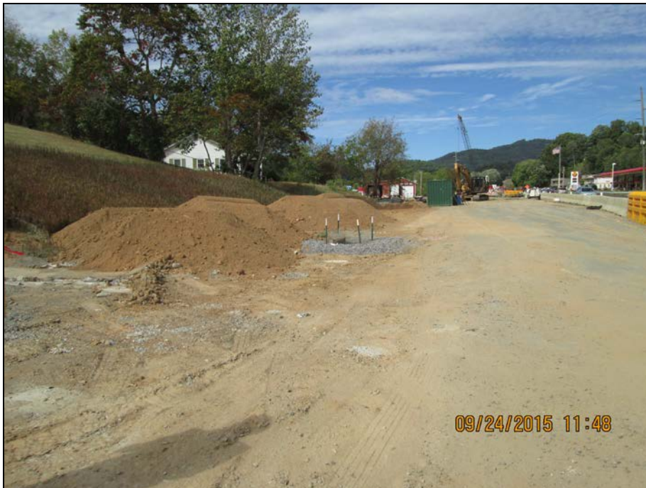
Several stockpiles were located less than 50 ft from surface inlets.
