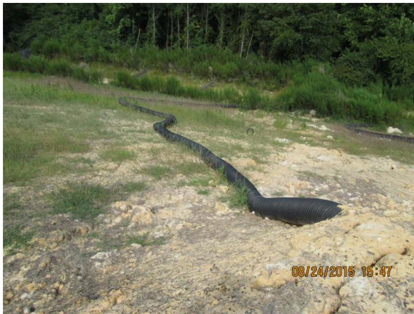
Temporary slope drain was not anchored well and the joints leaked contributed to deposition at the silt fence.
