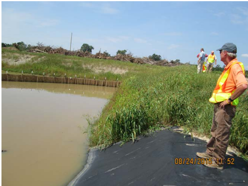
Temporary groundcover establishment is underway on this newly constructed temporary skimmer basin.
