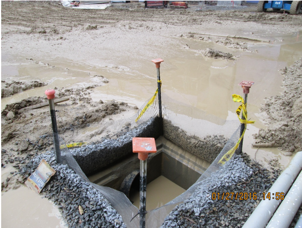
Site 1 - Revised plan needed to address additional sediment control needs at inlet draining offsite.
