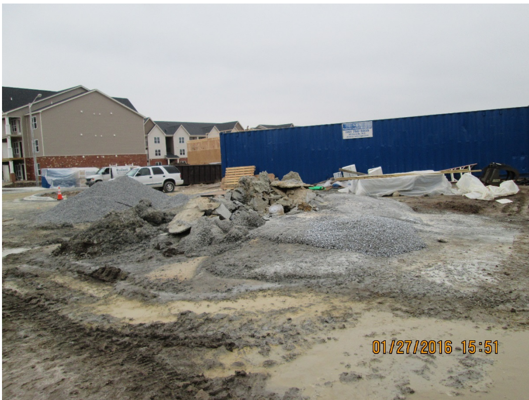
Site 2 – Concrete washout area needed for site.
