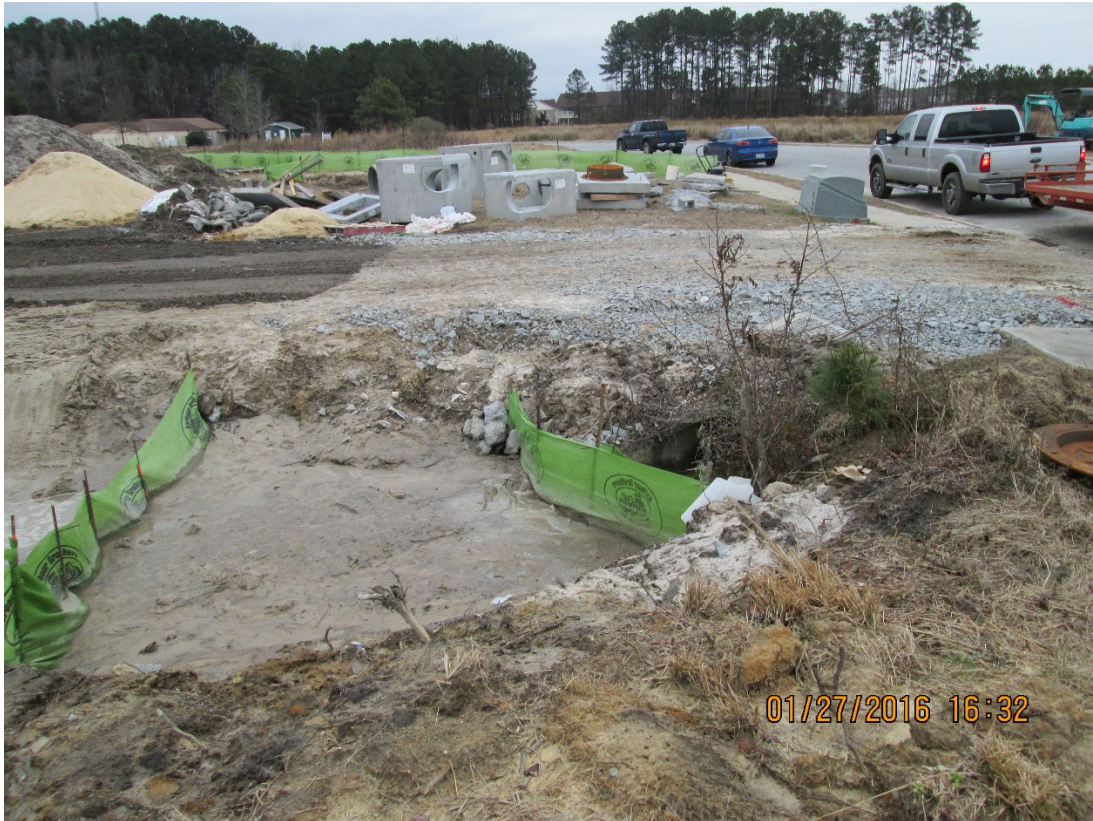
Site 3 – Revised plan needed to address additional sediment control for culvert that drains offsite.
