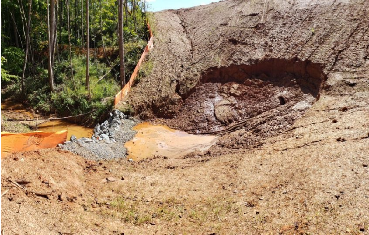
Photo- Previously taken photo from slope failure and sediment loss (NCDOT staff provided)
