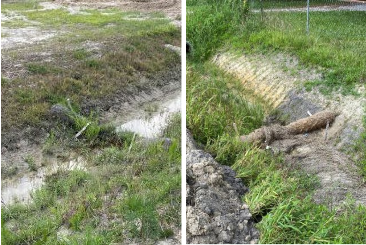
Photo- Wattles needing repair or replacement
