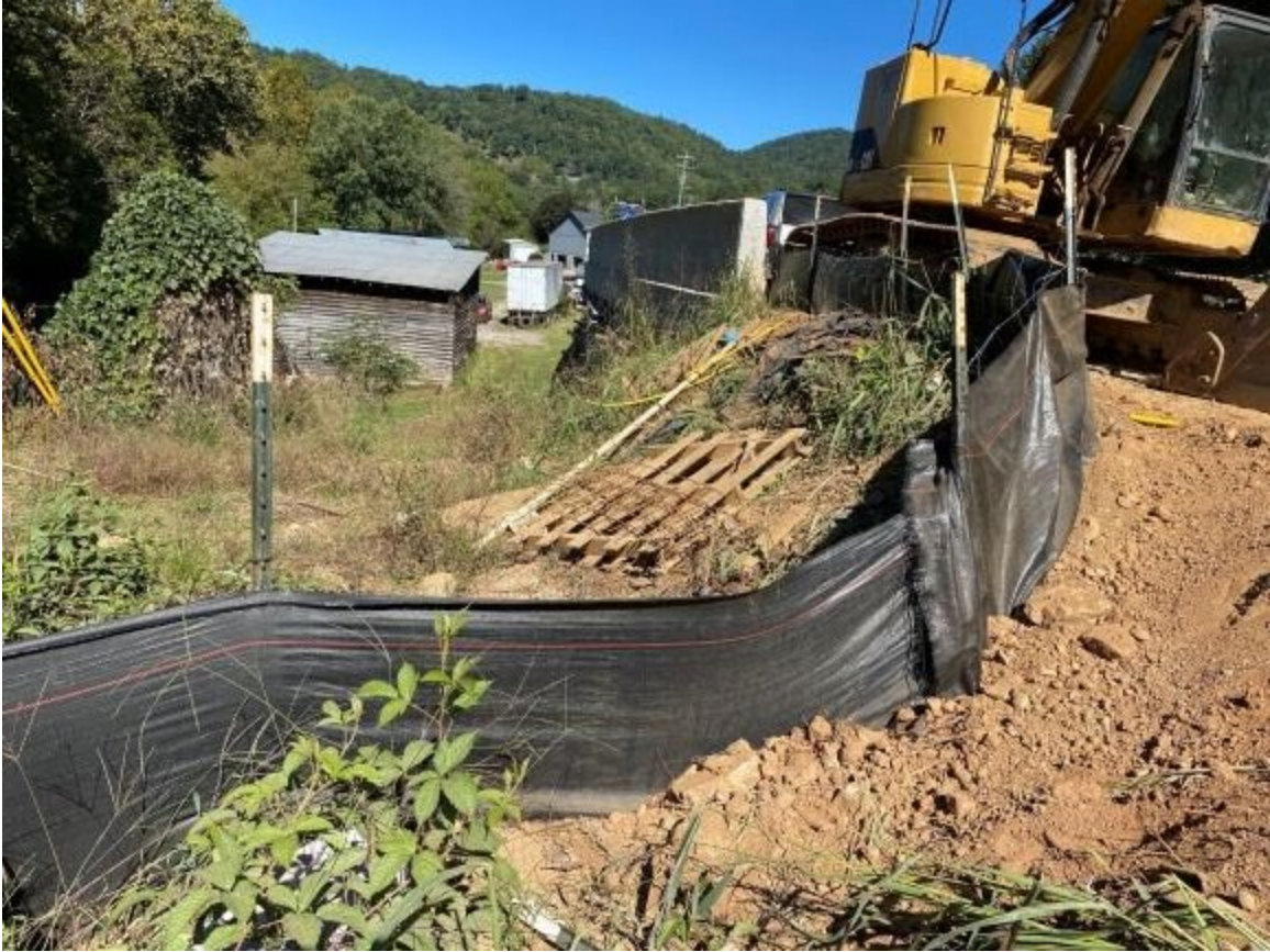
Photo- Materials placed outside of the silt fence
