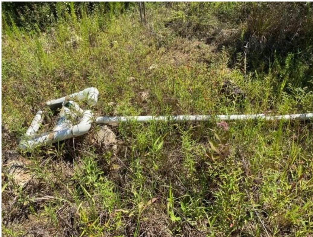
Photo- Skimmer not attached at Borrow Pit site
