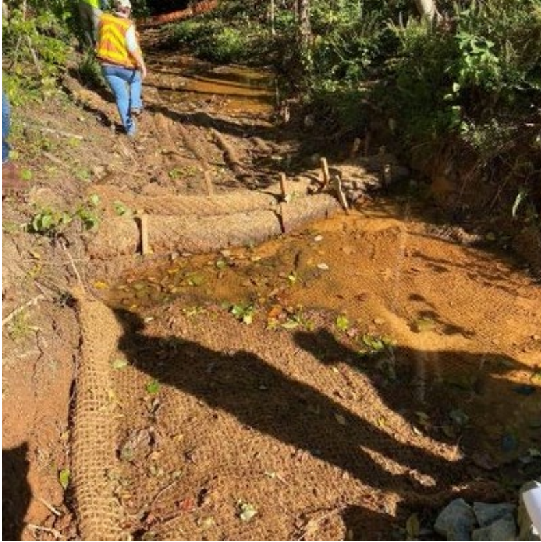
Photo- Signs of sediment loss and repairs in stream
