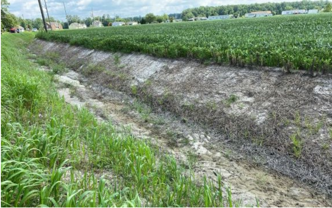
Photo- Ditch slopes needing stabilization
