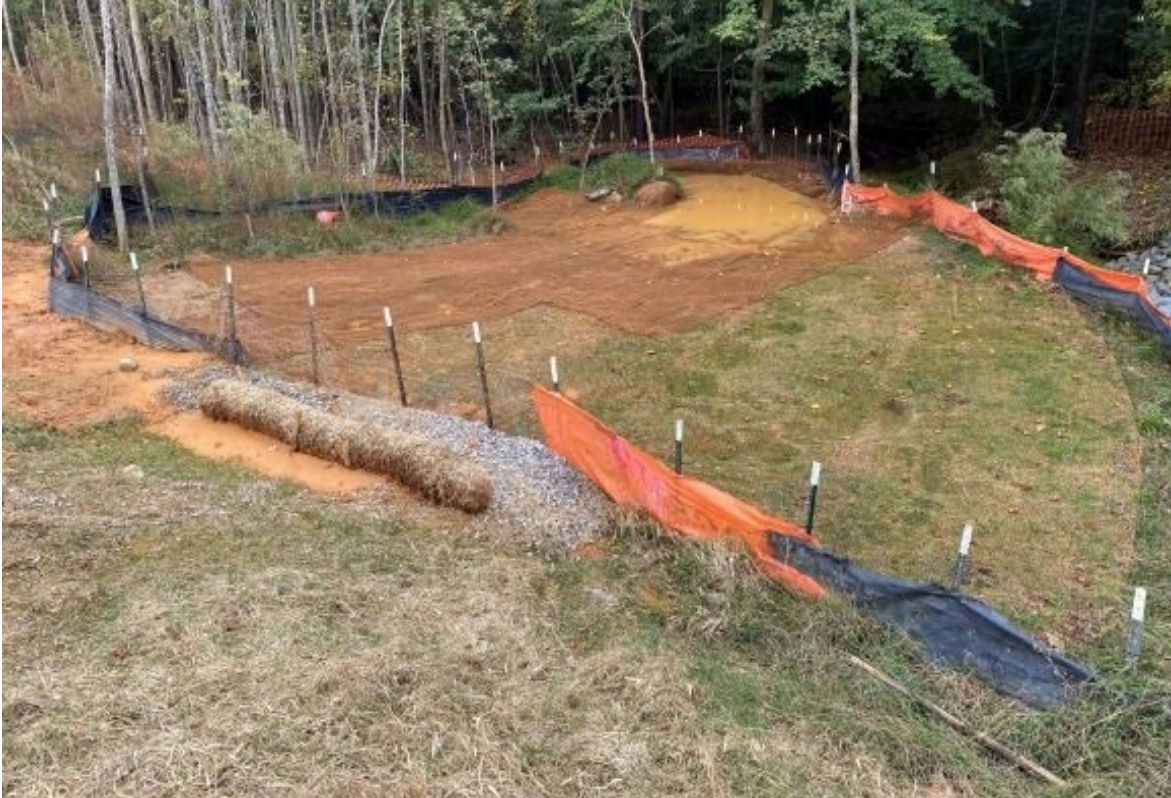
Photo- Area previously repaired
