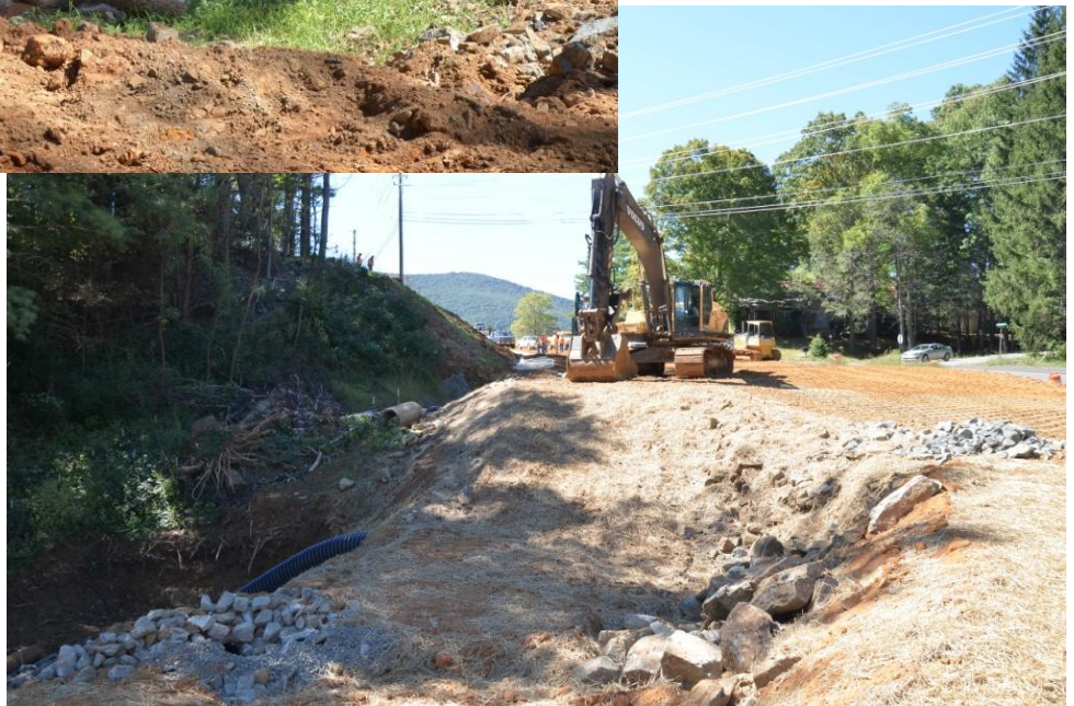
NC 88, Jefferson—Skimmer Sediment Basin discharges through land clearing debris down unstable excavated slope and into pond.
