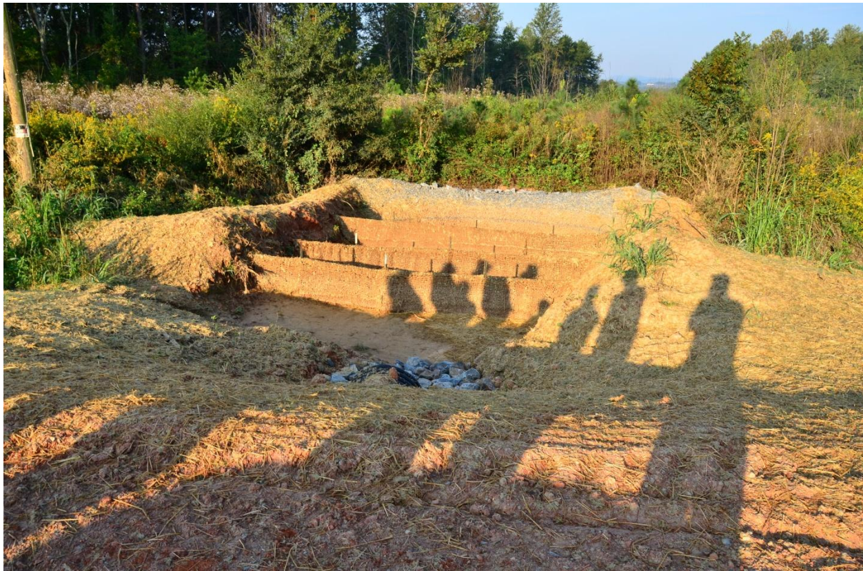
Willis Road, SR 1644 Silt Basin Type B with 8.5 acre drainage area.
