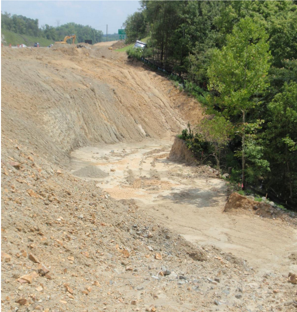
Fill slope with two rows of silt fence on creek bank on I-485 Design Build project.
