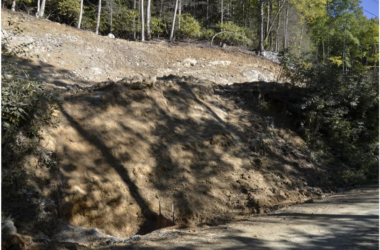
Fill slope above culvert inlet on Laurel Creek Road, SR 1123, Watauga County
