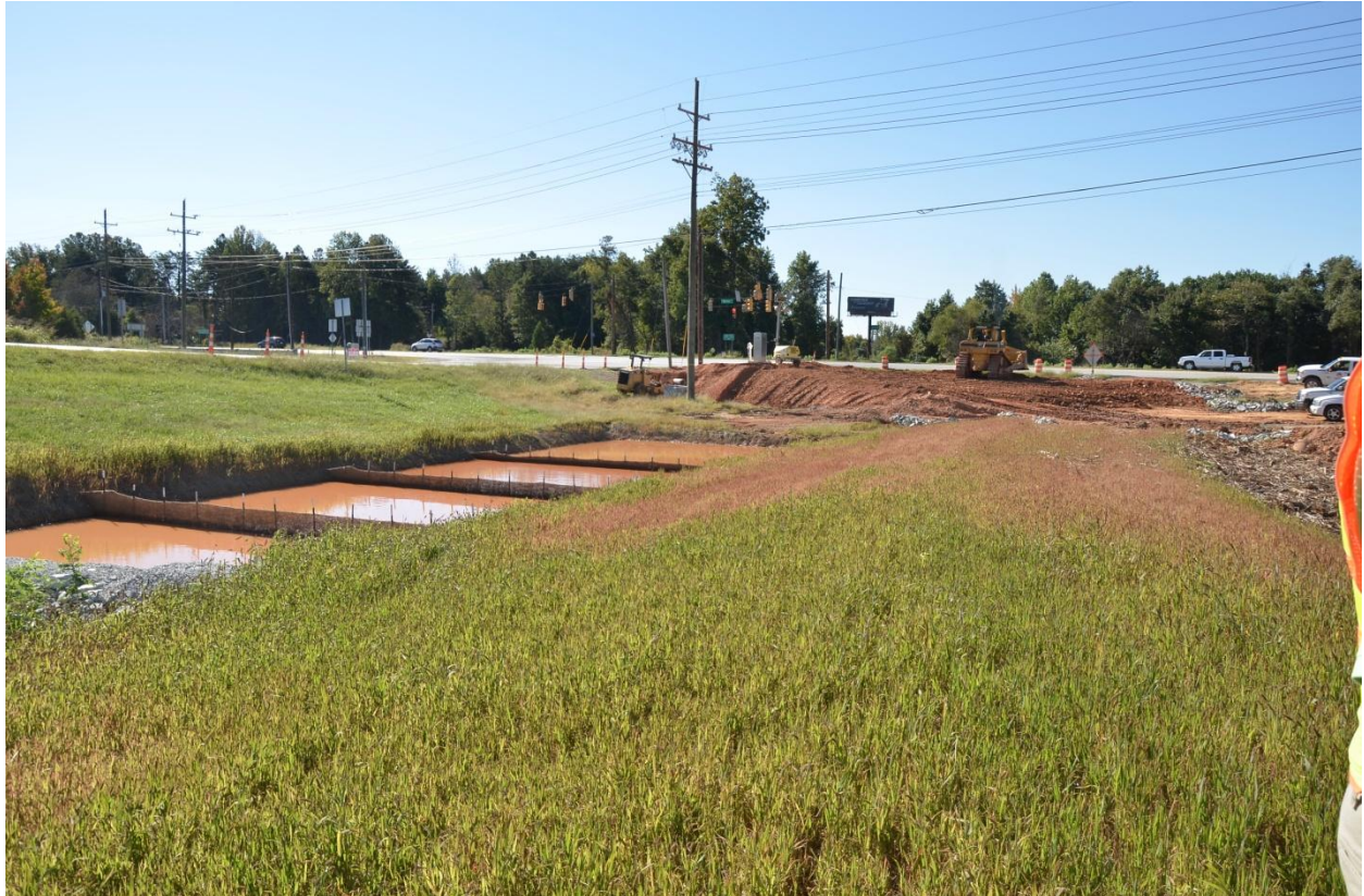
Temporary Rock Sediment Dam-Type B on West Market Street, SR 1008
