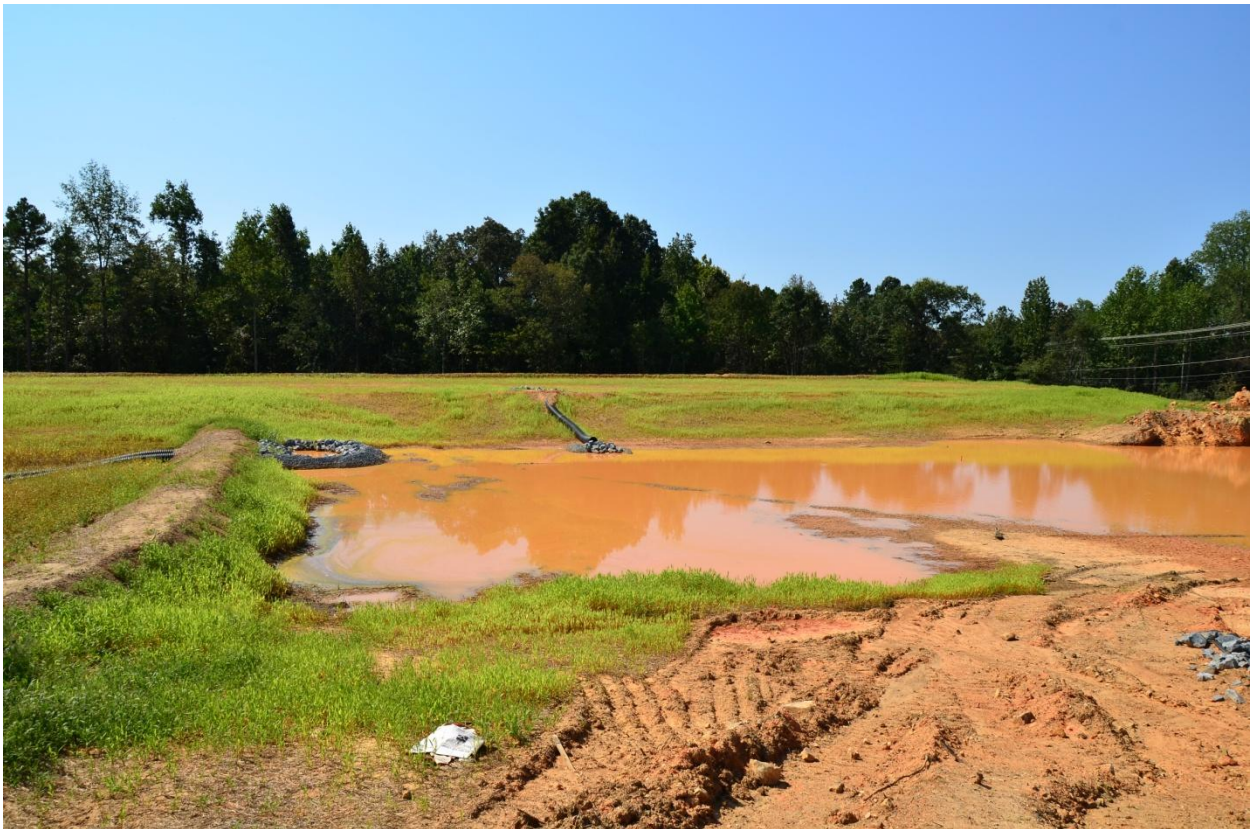
I-485 basin for 9 acre drainage area without surface dewatering or porous baffles
