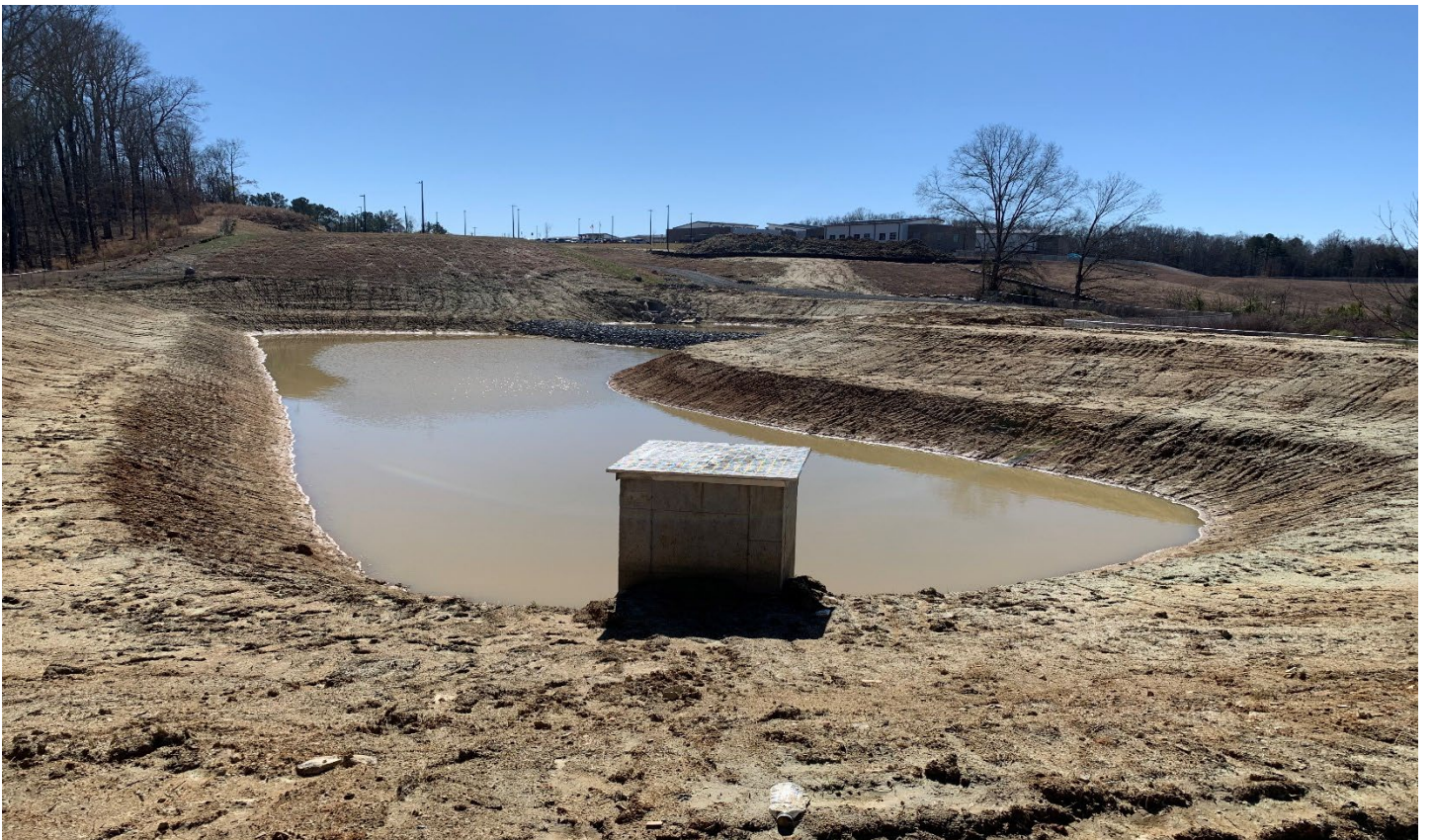
Picture #2: 03/03/2021 Sediment Basin Condition.
