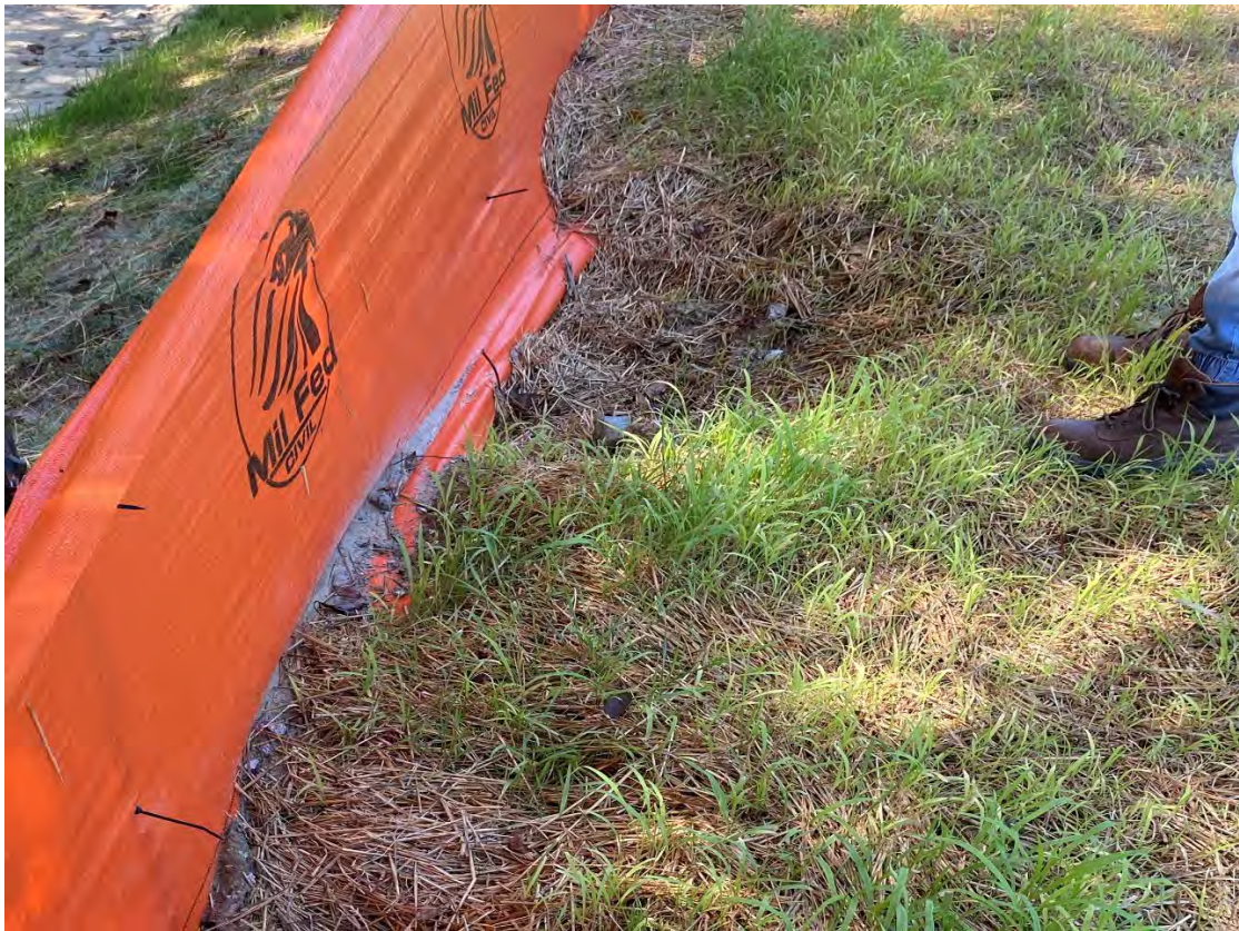
Silt fence undermined
