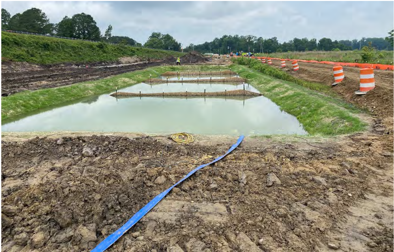
Skimmer device not installed, and diversion ditch not yet tied into basin
