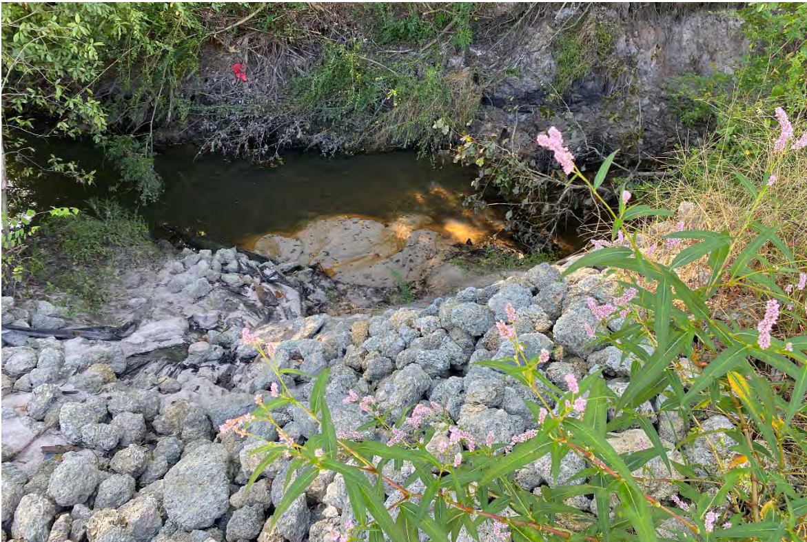
Sediment loss into stream
