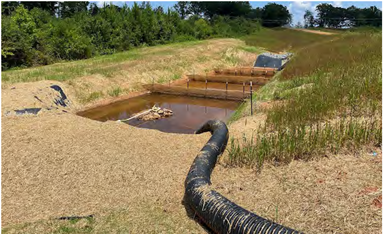
Slope drains placed in the wrong bay of skimmer basins
