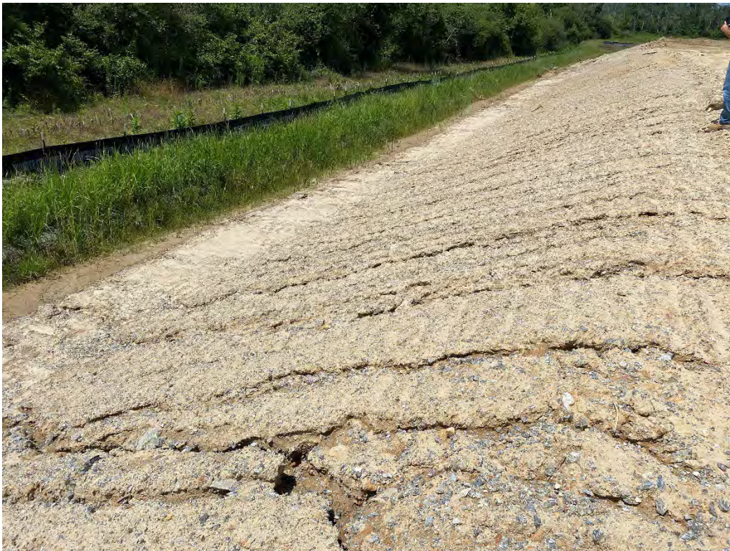
Rills formed on waste site slopes needing repair and stabilization
