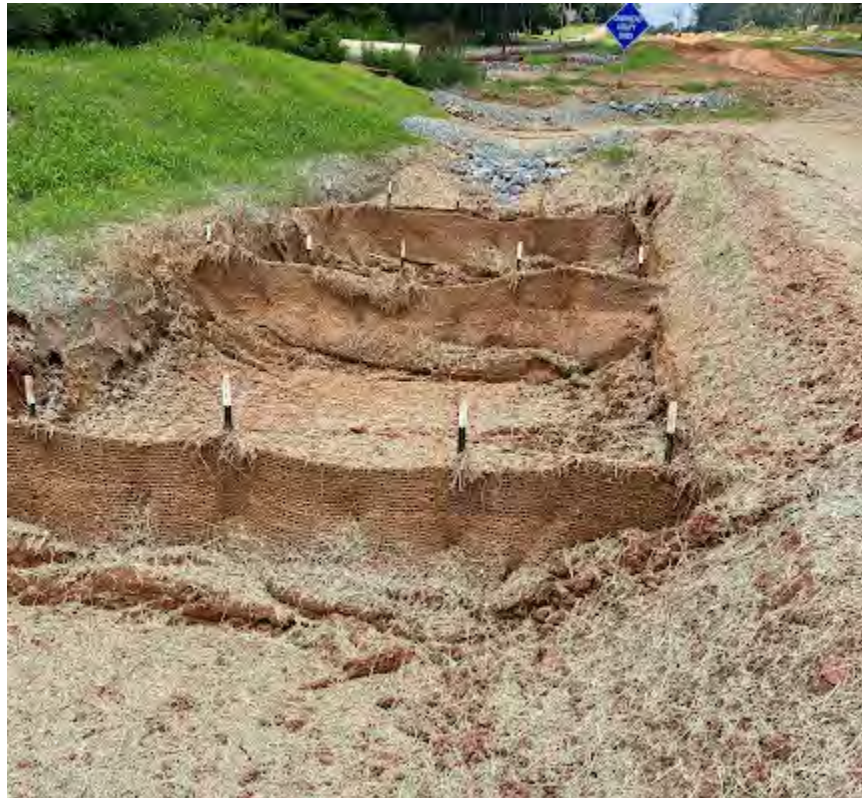
Sediment trap recently mucked out
