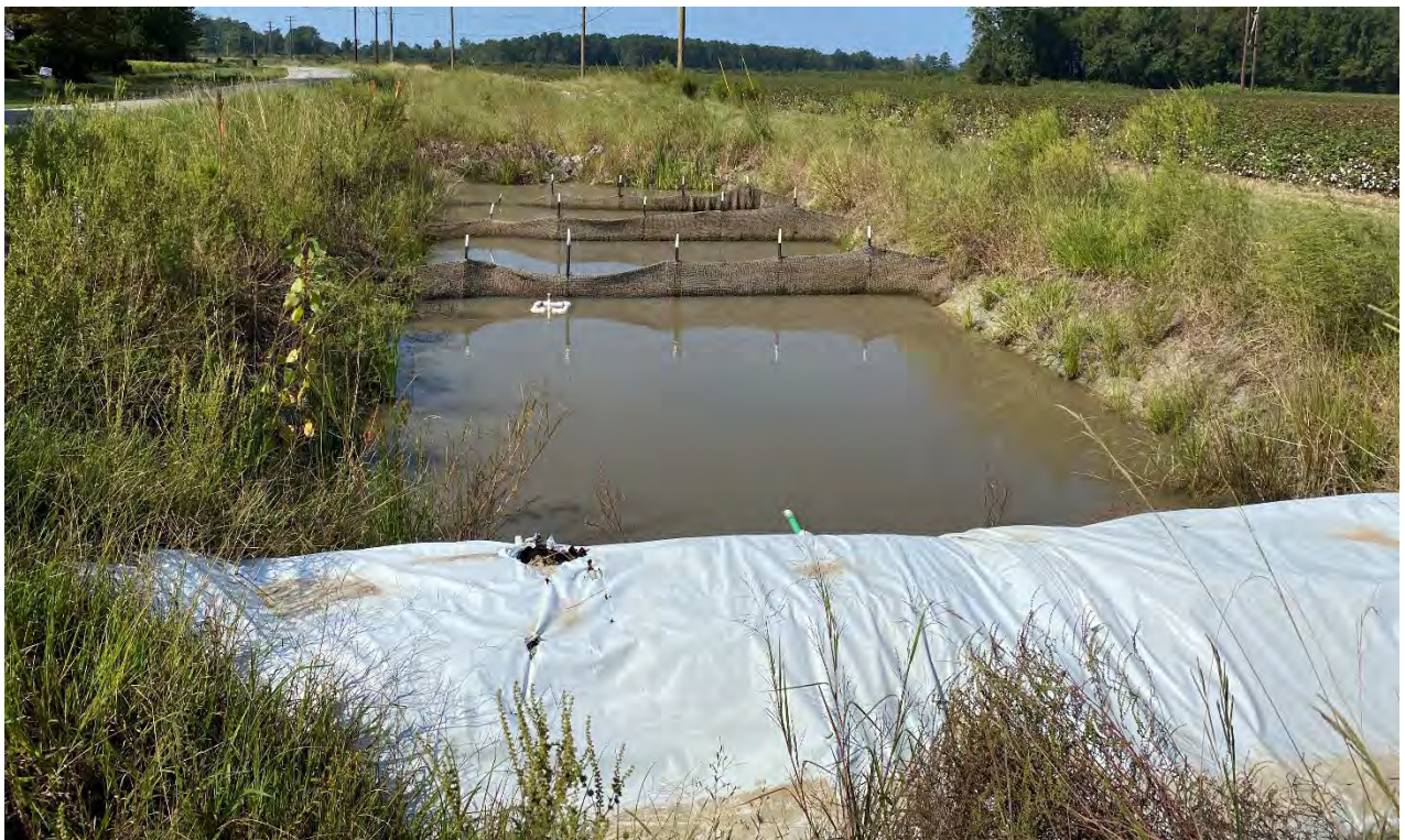
Skimmer device detached and spillway liner damaged
