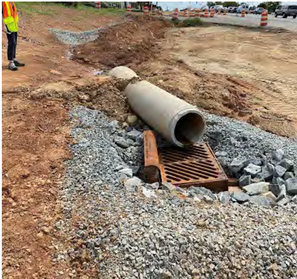
Pipe placed to convey flow from water leak
