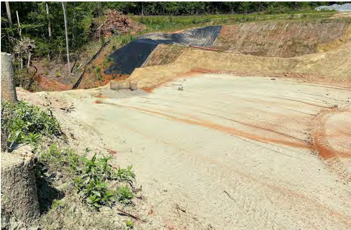
Basin and drop inlet protection measure
