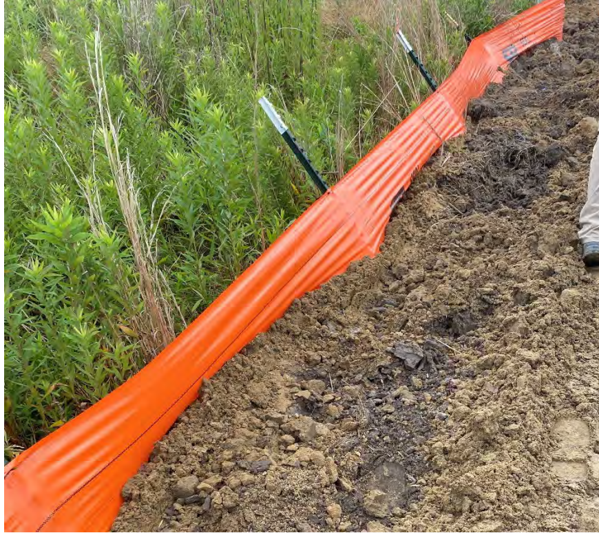
Silt fence being pushed over
