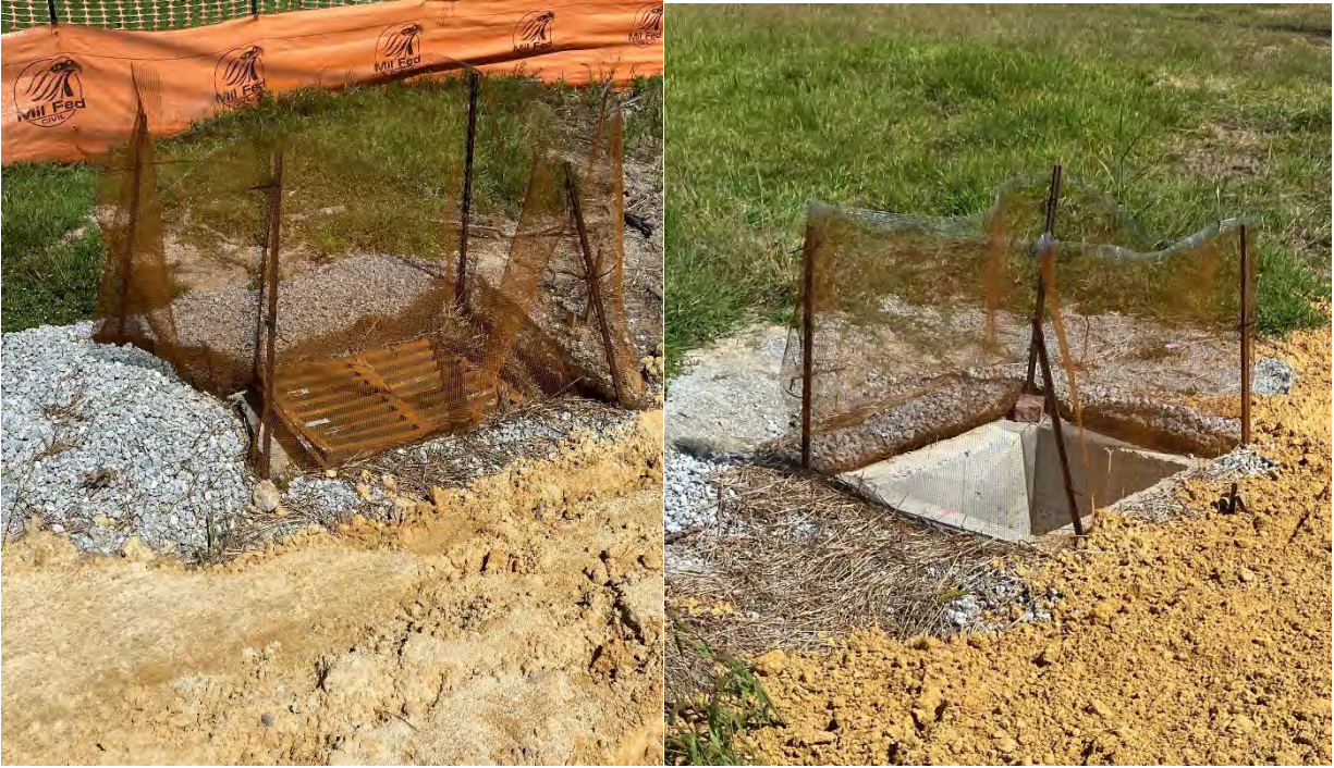
Drop inlet protection measures needing maintenance
