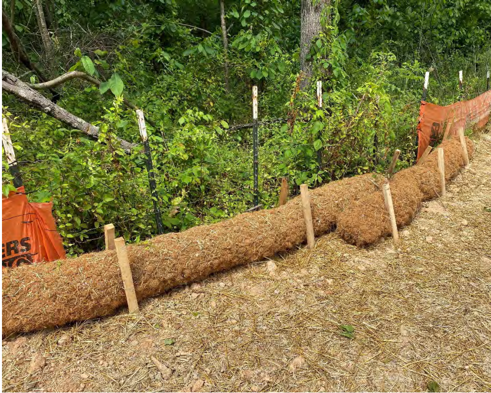
Silt fence wattle break
