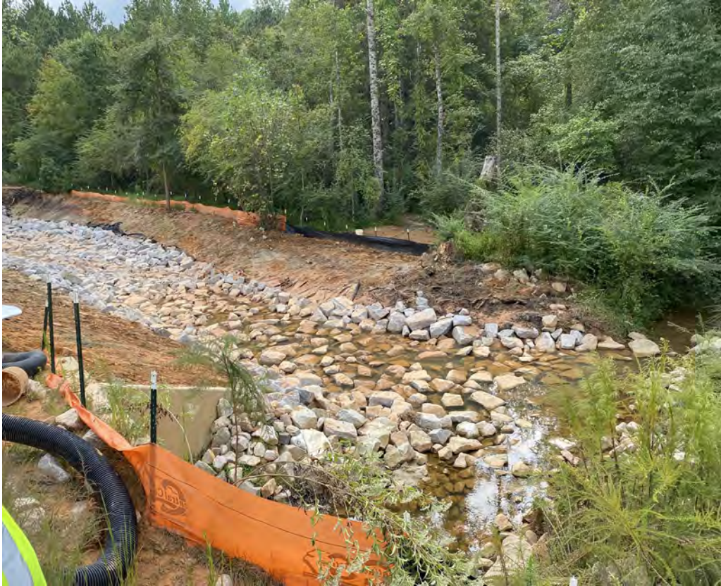
Channel adjacent previously noted sediment loss
