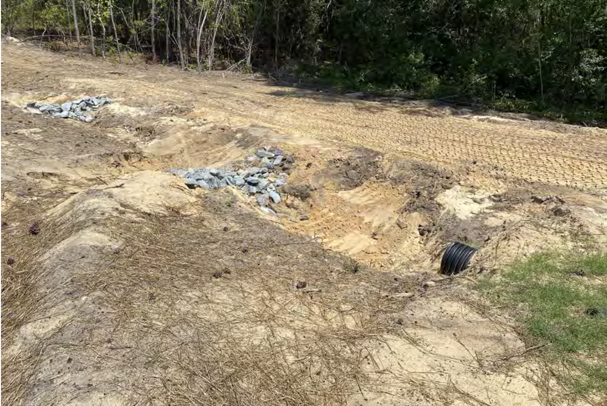
Silt fence removed and needing to be reinstalled
