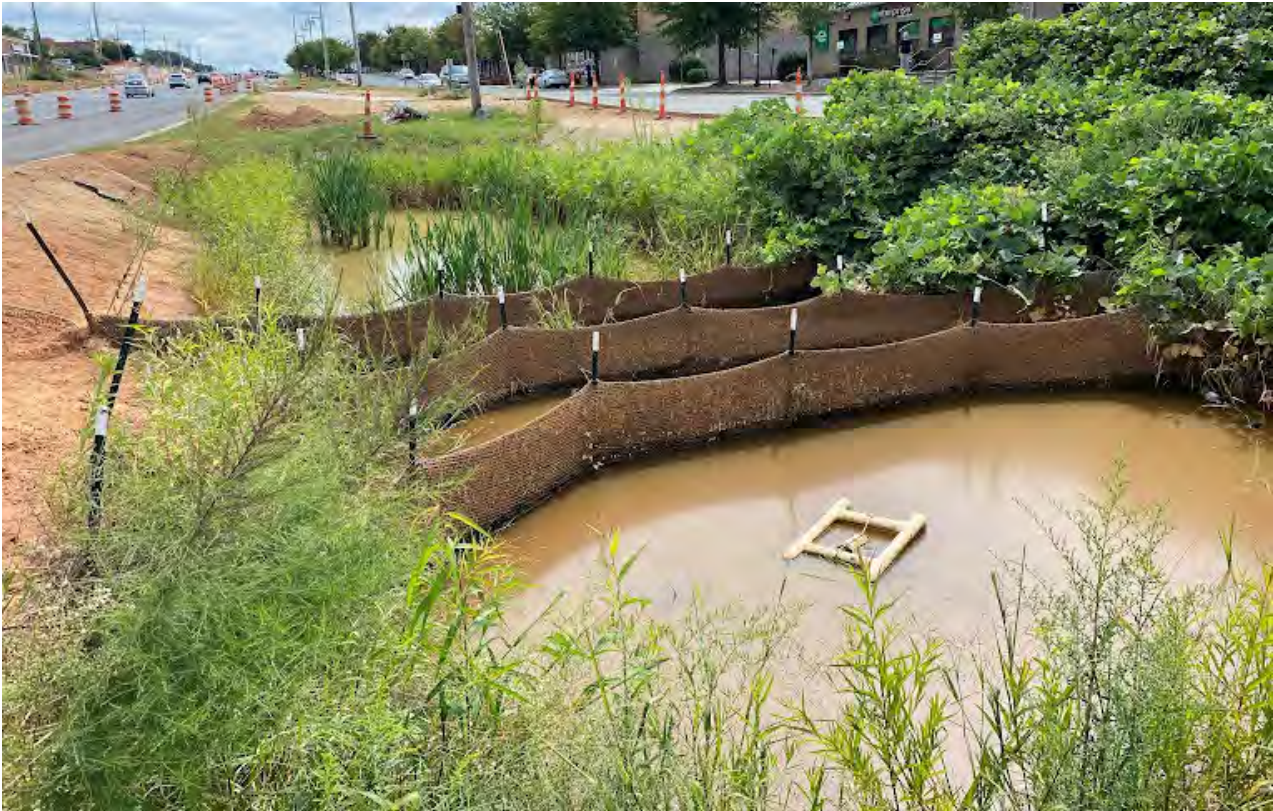
Baffles not properly spaced
