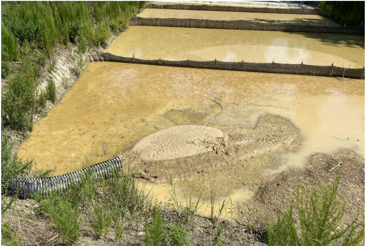
Skimmer basin on waste site
