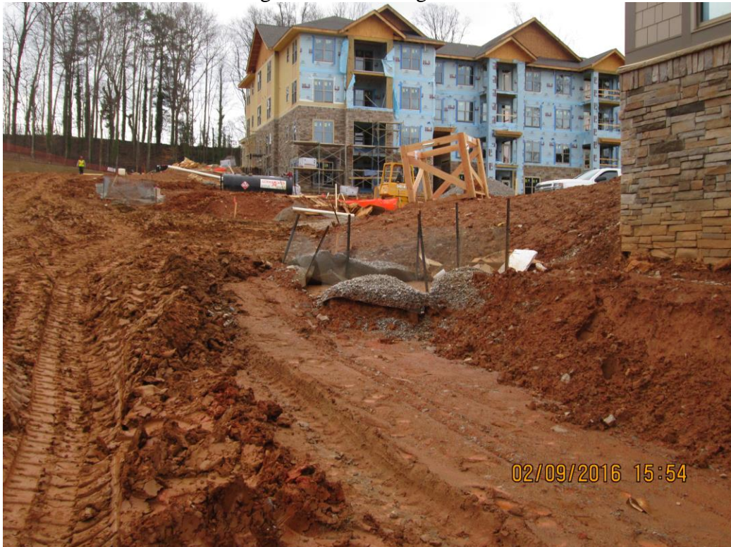
Site 2 - Inlet protection needs to be maintained.
