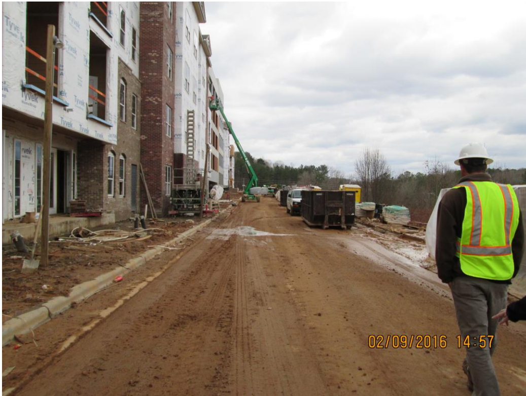
Site 1 – Mud in streets onsite leading to some tracking on offsite street.
