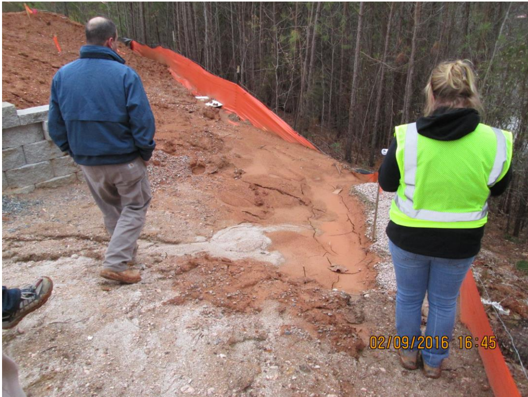
Site 3 – Perimeter silt fence needs maintenance adjacent to retaining wall.
