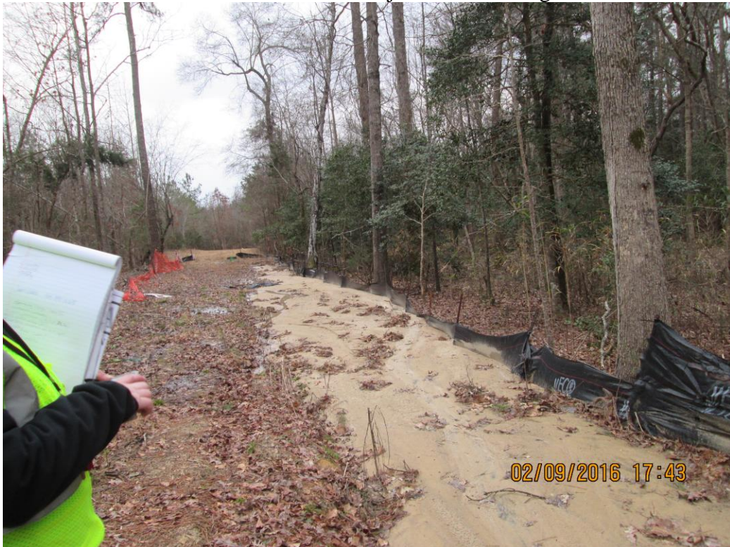
Site 4 – Perimeter silt fence needs maintenance along sanitary sewer easement.
