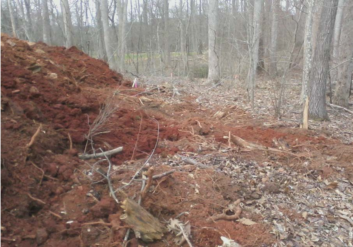
Site 3 – Silt fence was supposed to be installed prior to fill placement near stream buffer.
