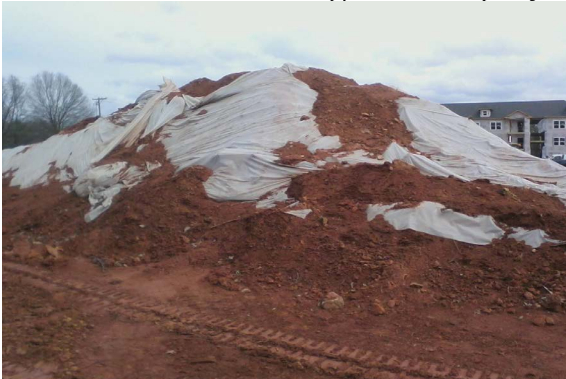
Site 2 – Stockpile has inadequate groundcover.
