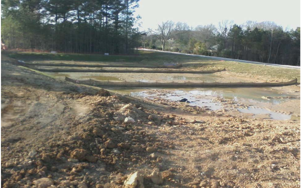
Site 5 – Temporary skimmer basin to be converted to permanent Stormwater BMP nearer the end of construction.
