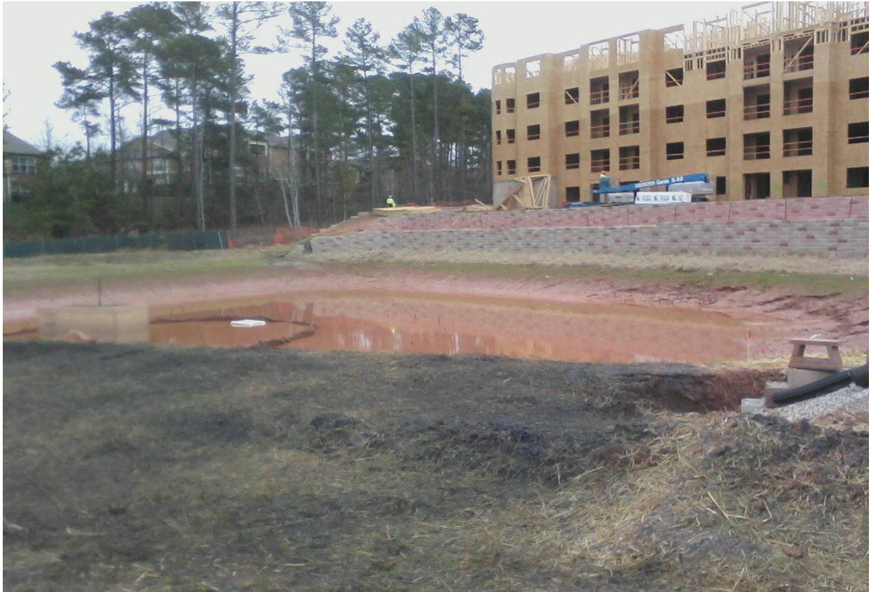
Site 3 – Temporary Skimmer Basin downstream of apartment building.
