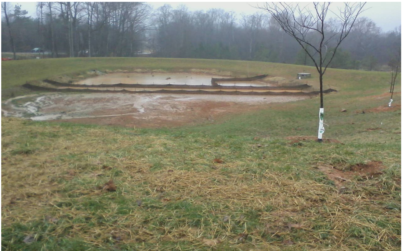
Site 2 – Good stabilization on temporary skimmer basin to be converted to permanent Stormwater BMP.
