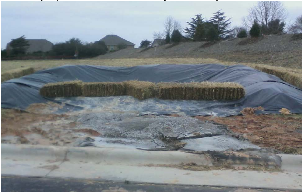
Site 4 – Improperly installed concrete washout area.
