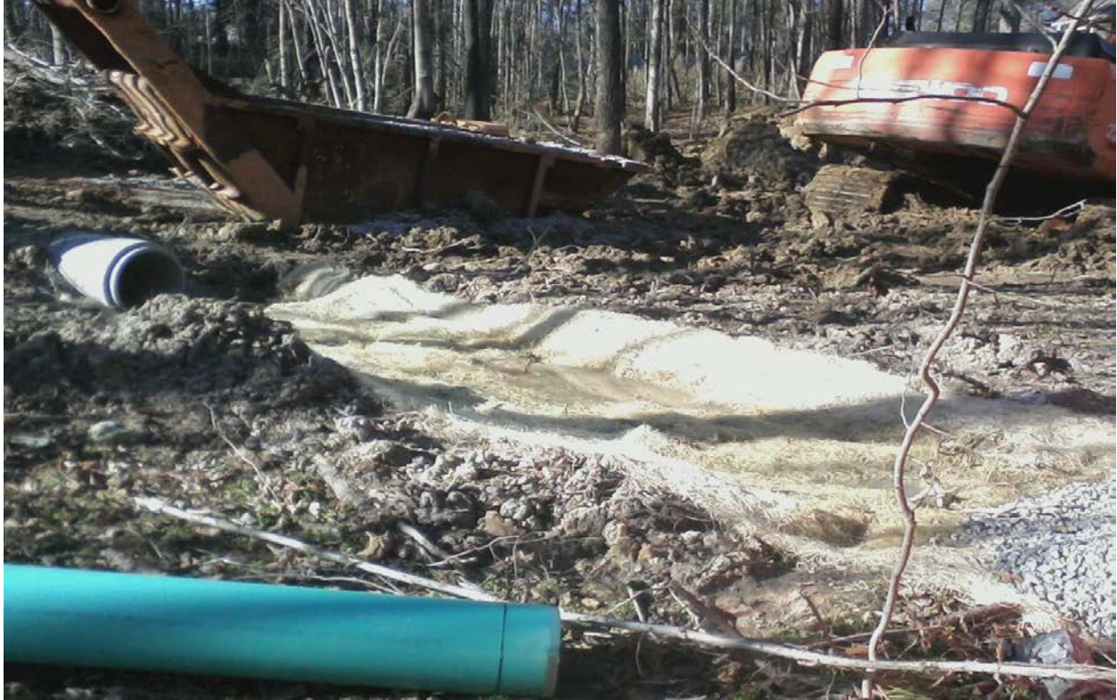
Site 3 – Temporary Skimmer Basin downstream of apartment building.
