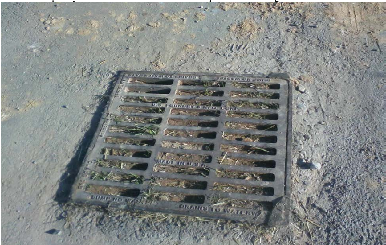
Site 4 – Inlet shows continued lack of maintenance with grass actively growing.
