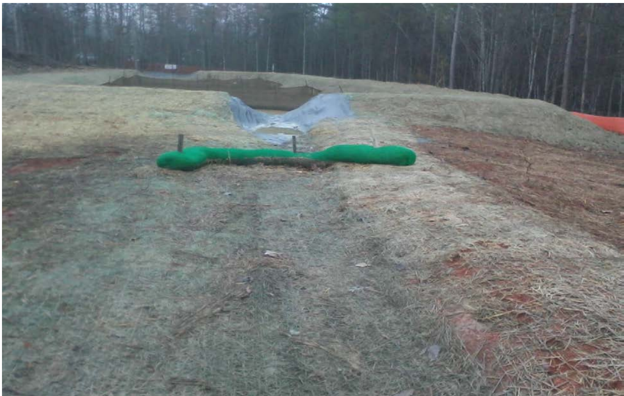
Site 4 – Perimeter controls have been stabilized or seeded and provided with mulch or rolled erosion control product.
