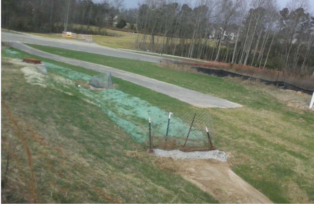
Site 1 – Check dam with lined channel
