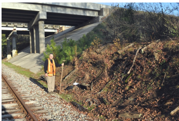
Figure 32b. Bethany Church outcrop is in poor condition in December 2010 showing locations of both bridge footings for US421. The newer eastbound bridge over US421 is in the foreground and the concrete apron has covered important parts of the original outcrop. Photograph taken in December 2010.
