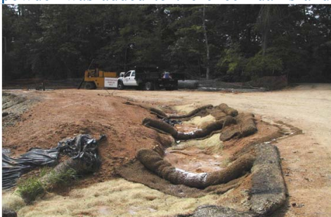
Figure 3. New entrance road with stabilized ditch (lining, fiber check dams) and PAM added to control turbidity..
