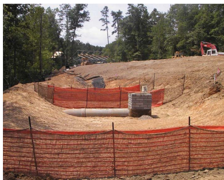
Figure 1. Skimmer basin now converted to constructed wetland with a bottom outlet (see stone at bottom of riser). Note inlet protection and wattles on the ditch at the far end.
