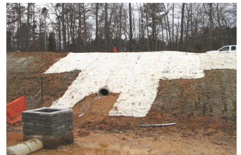
Figure 4. Stabilization of the basin slope with erosion control blankets. Note the coir matting installed below the pipe outlet to prevent scour and for PAM powder application..
