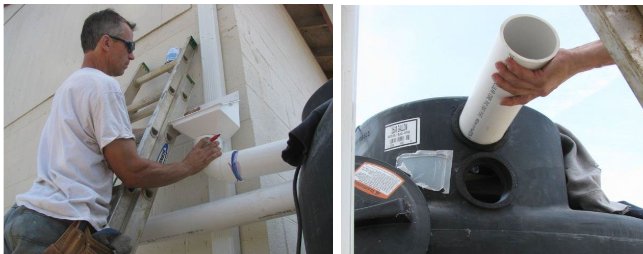
Figure 14. (a) Pipe leading from debris filter to the tank; (b) Rubber gasket used to create leak-free seal when pipe enters the tank. (NCSU-BAE)
