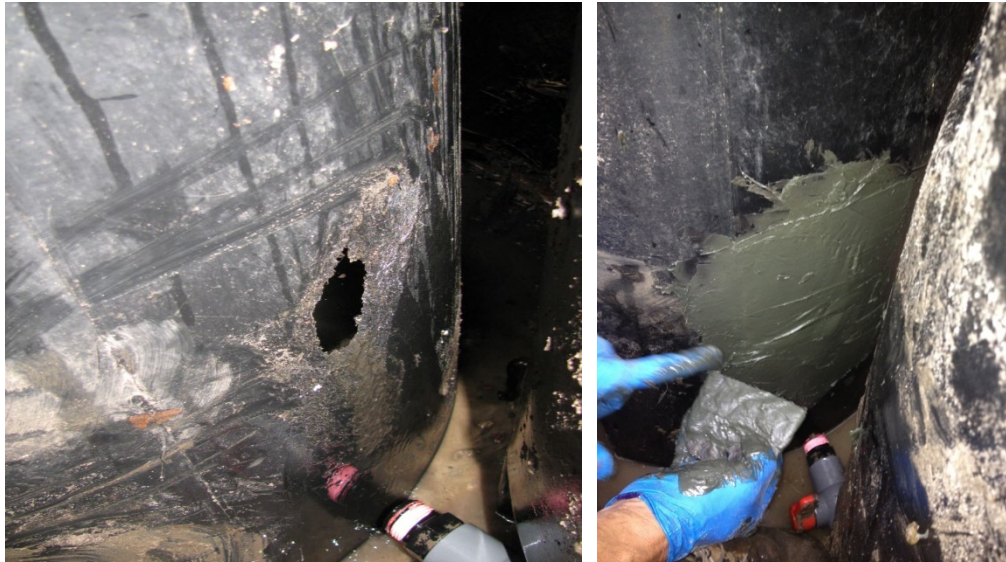
Figure 16. Example of animal damage to cistern and patching of hole. (NCSU BAE)
