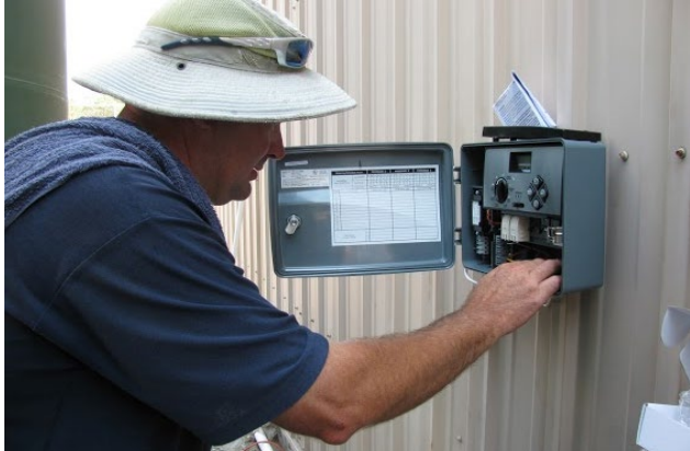
Figure 8. Irrigation Controller (NCSU BAE)
