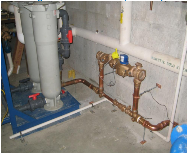
Figure 9. Water Meter (UNC-CH)
