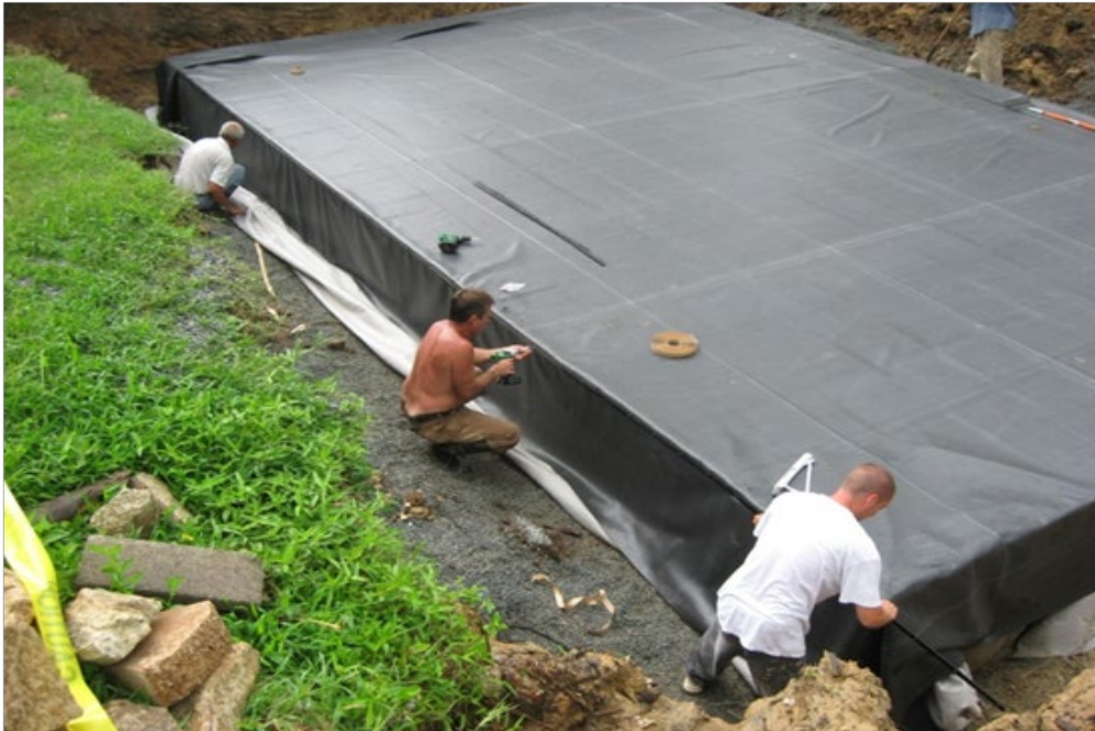
Figure 12. Installation of a membrane on a 15,000 gallon underground cistern at the Fayetteville Technical Community College NCSU BAE)
