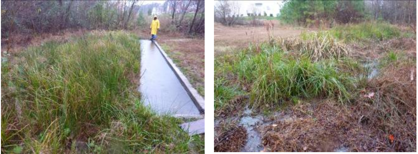
Figure 13: Unmaintained Blind Swale and Unmown FS
