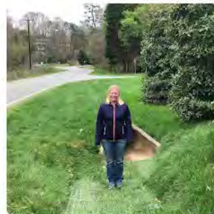
Regents Park Rd and Finborough Ct - ScourStop 6 items - Shared
