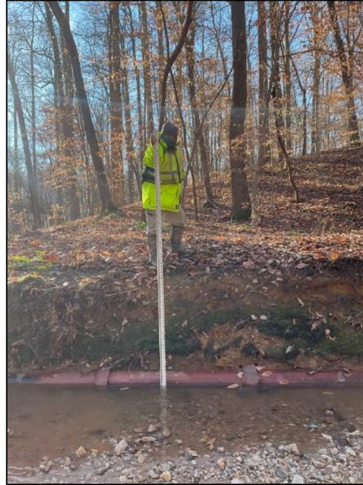
Exposed sewer line Walnut Creek Trib Adj Ivy Ln Cary, NC
