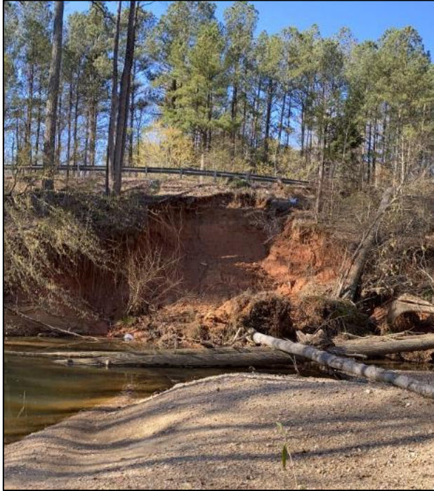
Bank collapse near hwy Richland Creek, Raleigh, NC
