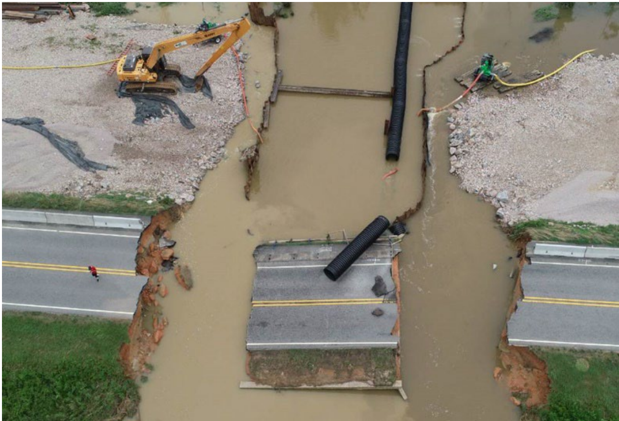
US 401 washout, Franklin County
