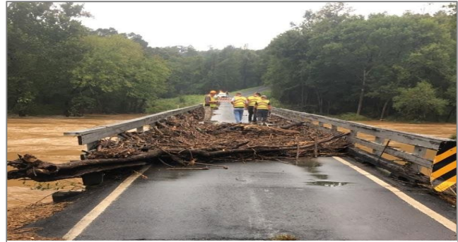
Flood damage along Bethlehem Church Road in Stanly County
