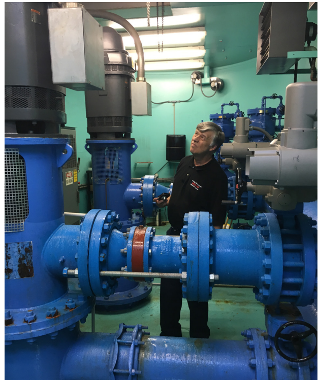
WRP engineer, Ron Haynes surveys a pump station of the Water Resources Department of the City of Asheville.
