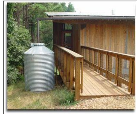
Cistern located at the Prairie Ridge education facility for the N.C. Museum of Natural Sciences is used to flush toilets within the facility.
