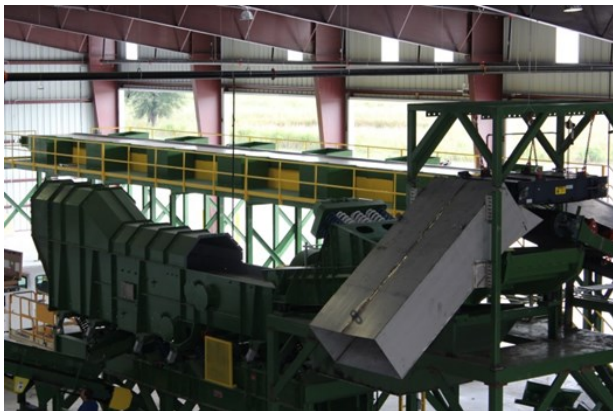
Green Recycling Solutions' multi-station pick-line is installed under roof and has the capacity to process approximately 300 tons per day.
