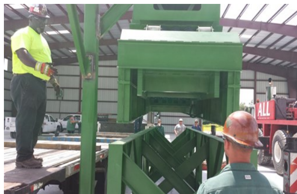
Workers install MetalTech System's state-of-the-art material processing equipment at Green Recycling Solutions' C&D recovery facility in Maysville.
