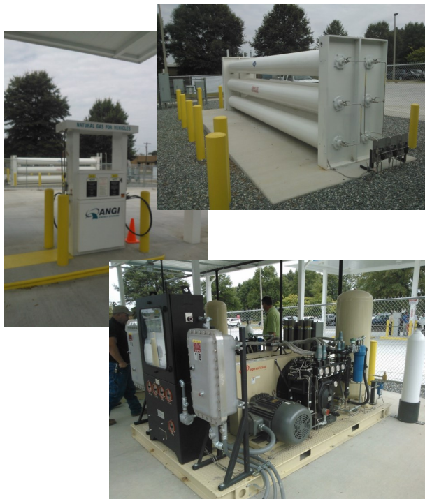
The three components of a fast-fill CNG station (shown clockwise above) include a three bank storage tank, a compressor, and a dispenser that operates much like a traditional gasoline filling station.
