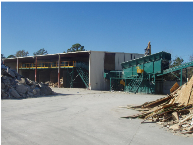
The Erin screening and sorting system pictured here is being installed at Griffin Brothers' Highway 49 facility near Harrisburg.
