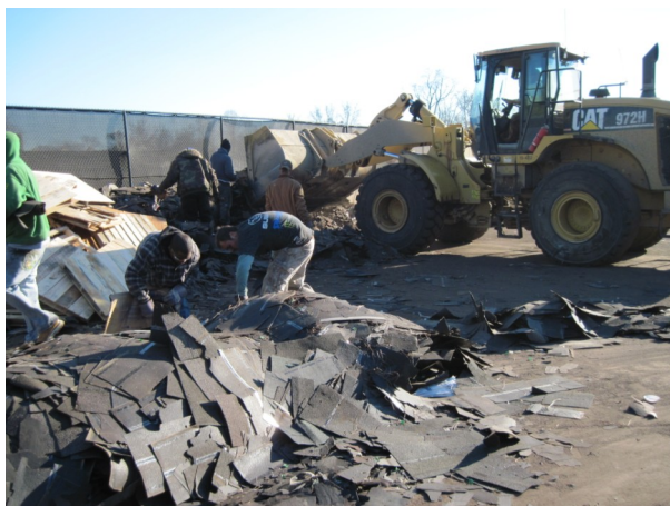
Workers clean up minor debris from an incoming asphalt shingle load at Boggs Paving, one of the conference tour sites.
