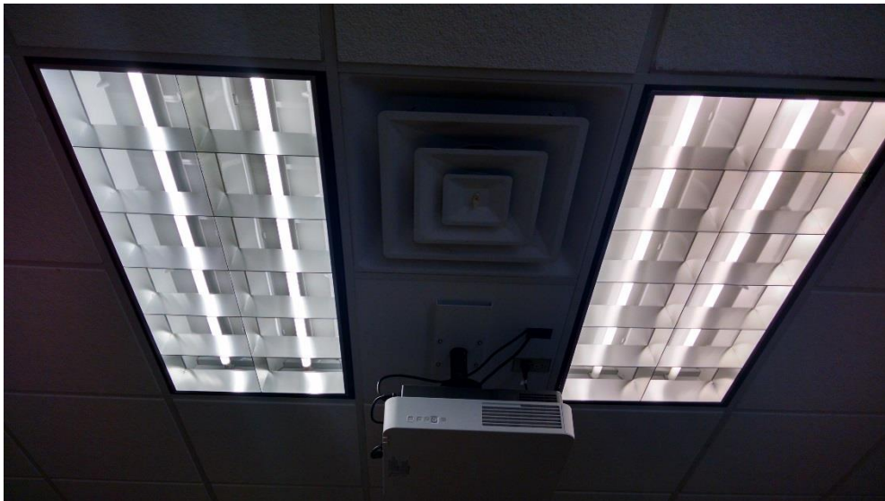
(2) 14 Watt LED with existing ballast
