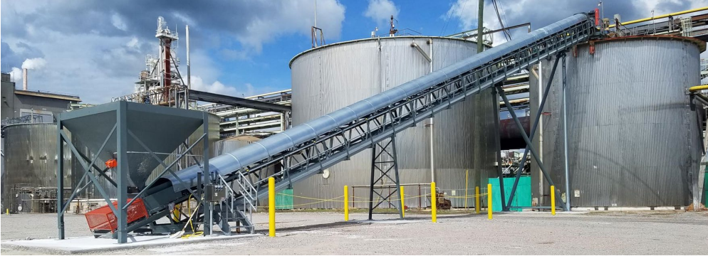
Hopper and Conveyor System
