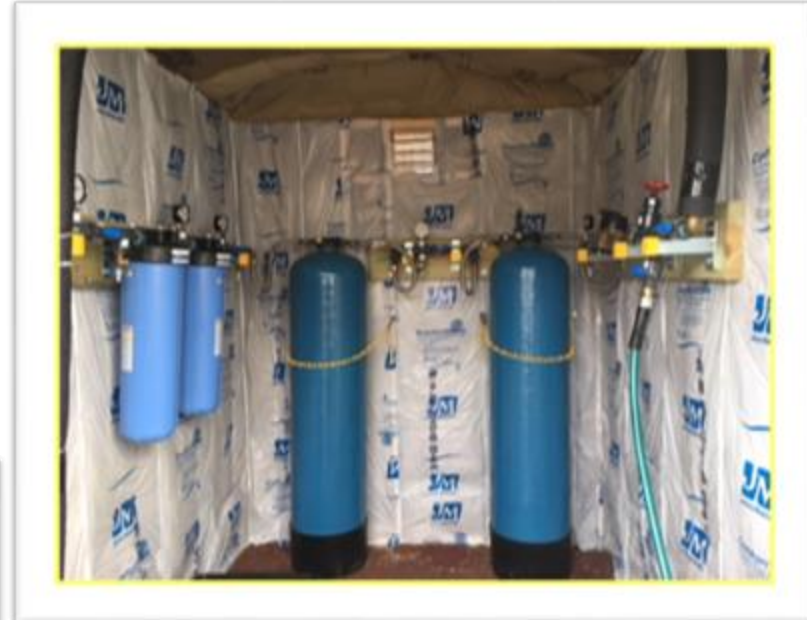
Whole-House Granular Activated Carbon system
