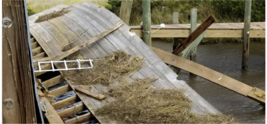
Damaged docks in Sea Level, North Carolina. Photo: North Carolina Fisheries Association
