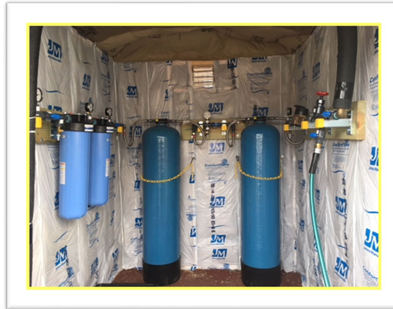
Whole-house Granular Activated Carbon system (left)
