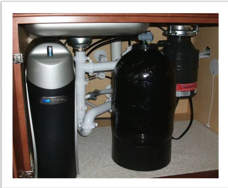
Reverse Osmosis System (right)
