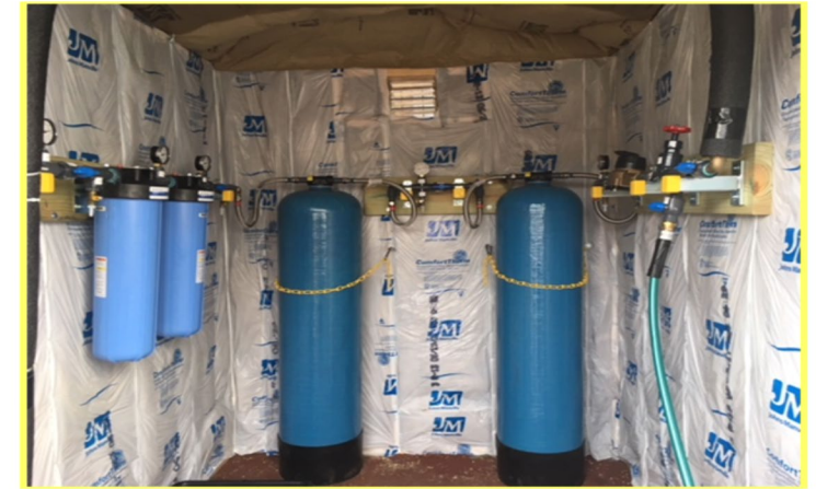
Whole house Granular Activated Carbon system
