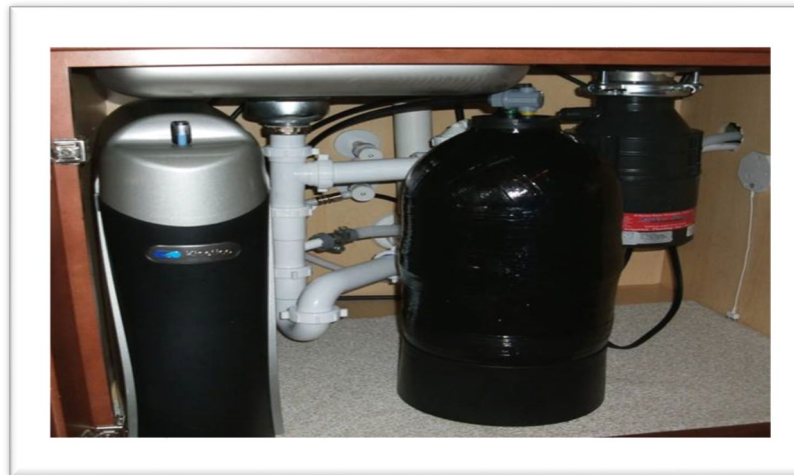
Reverse Osmosis System
