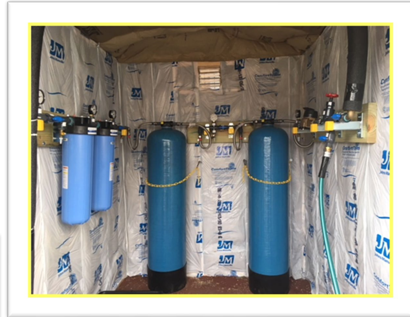
Whole-House Granular Activated Carbon system
