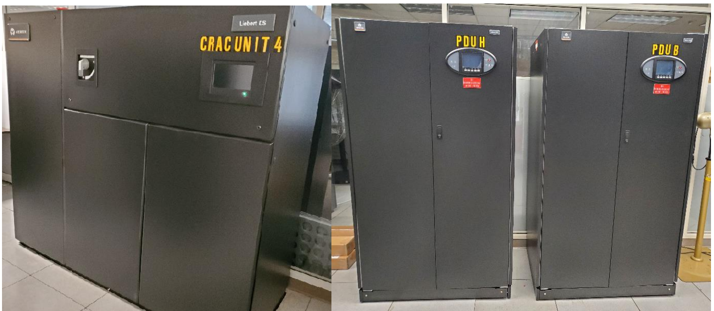
Newly installed equipment inside of our Data Center
