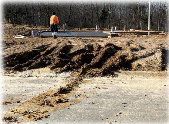
Figure 8 - Poor Construction Entrance
