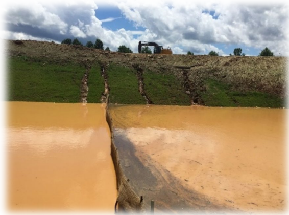
Figure 11 - Rill Erosion on Sediment Basin Slope
