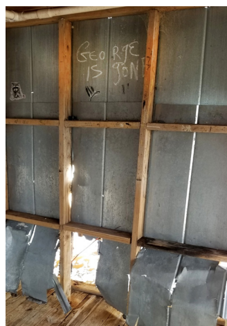
Fish house damage in Sea Level, North Carolina. Photo: North Carolina Fisheries Association
