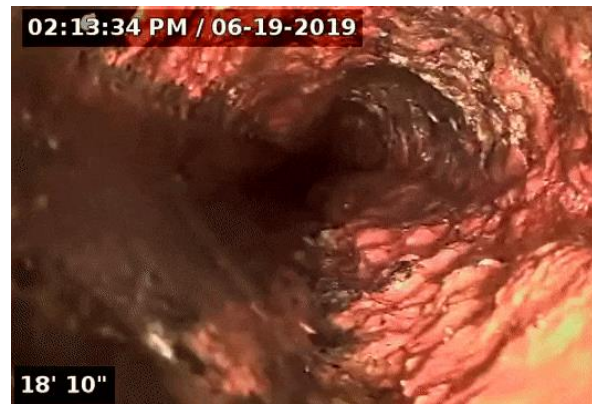
Grease, fat, oil buildup
