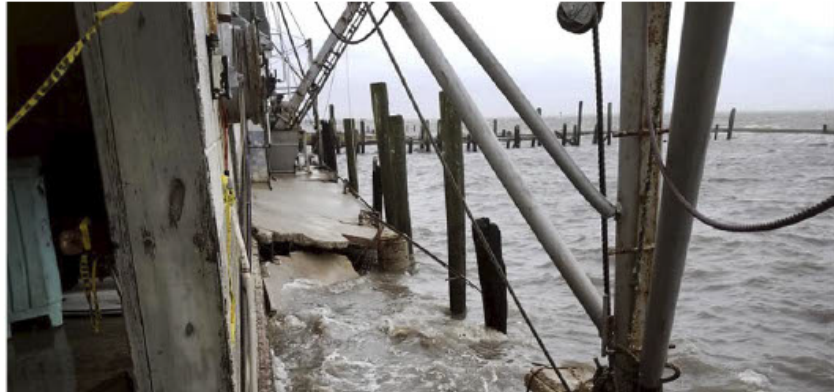
Damaged seafood processor/dealer. Photo: North Carolina Fisheries Association/Charles Smith
