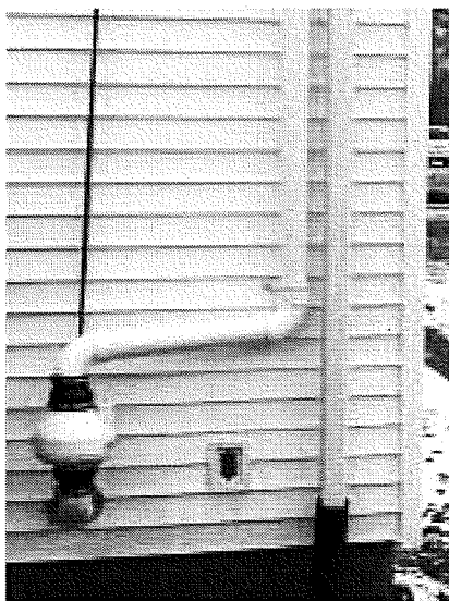
A subsurface depressurization system fan on the exterior of a building.
