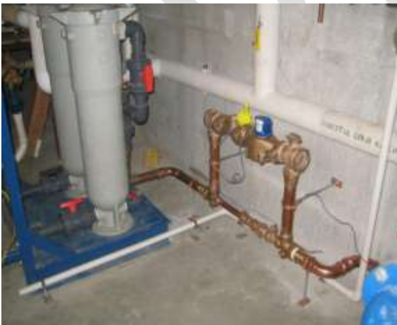
Figure 25-13. A water meter from the local public water/sewer provider is installed where harvested rainwater the building to be used for toilet flushing. (UNC-CH)
