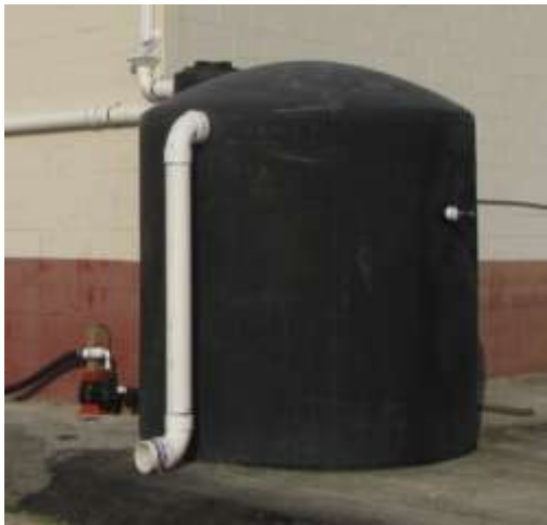
Figure 25-10. Example of an overflow at an NCDOT Facility (NCSU BAE)
