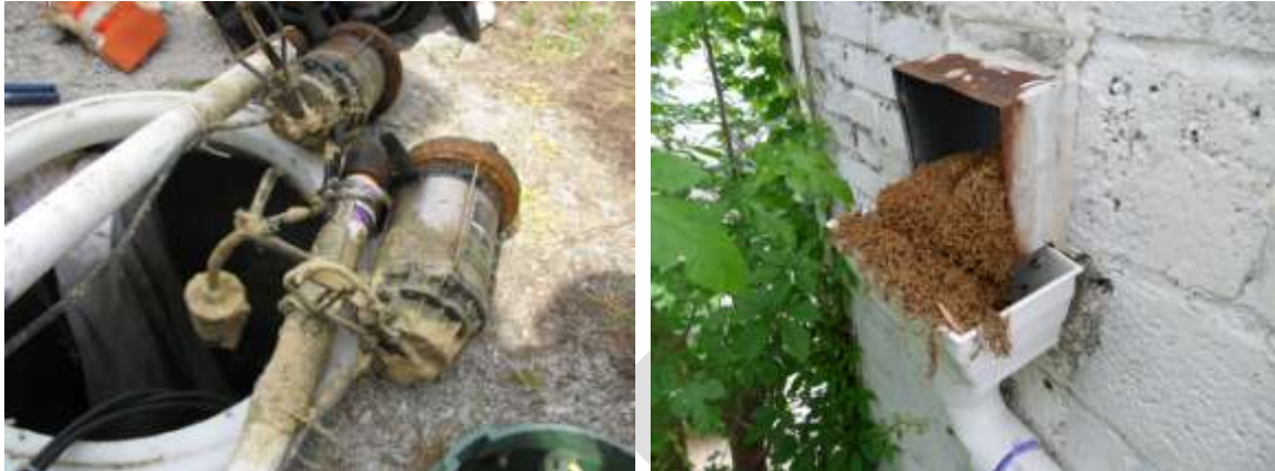
Figure 25-20. Pumps need to be pulled periodically for cleaning and preventive maintenance (left). Overhanging vegetation increases the needed frequency of maintenance (right) (NCSU BAE)
