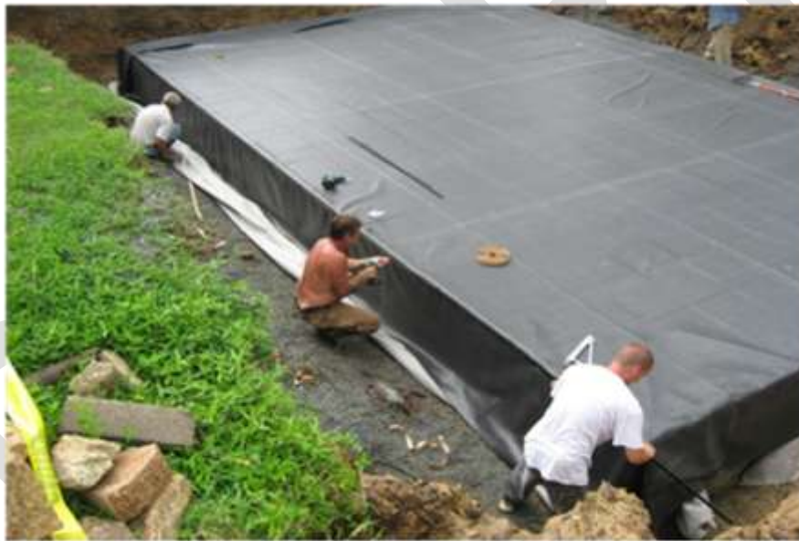
Figure 25-17. Installation of a membrane on a 15,000 gallon underground cistern at the Fayetteville Technical Community College NCSU BAE)
