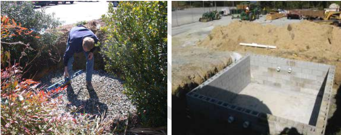
Figure 25-15. Preparing a cistern footing of aggregate (left) and a concrete footing for a cistern exceeding 1,500 gallons (right) (NCSU BAE)
