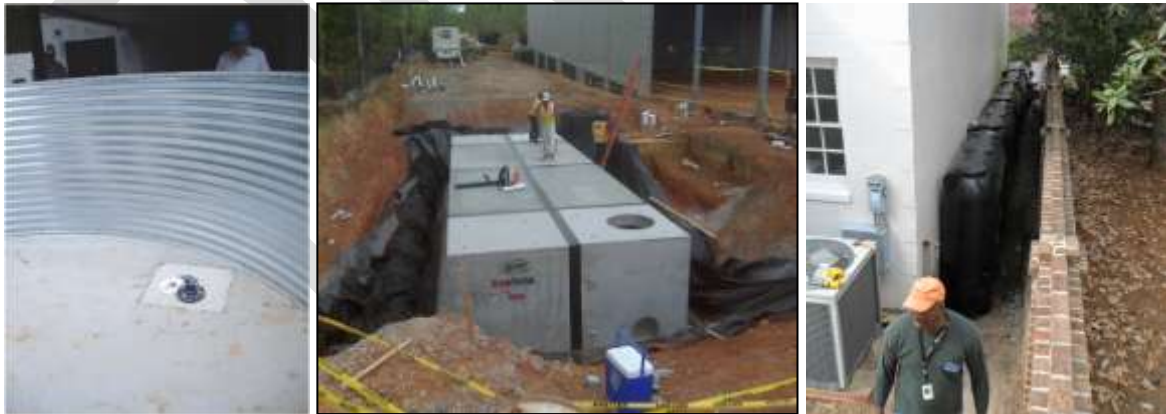
Figure 25-12. Metal cistern under construction (left), underground concrete vault wrapped in an impermeable liner (center) and a series of plastic cisterns (right) (UNC-CH left and NCSU BAE center and right)
