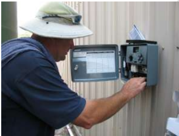
Figure 25-14. An Irrigation Controller (NCSU BAE)
