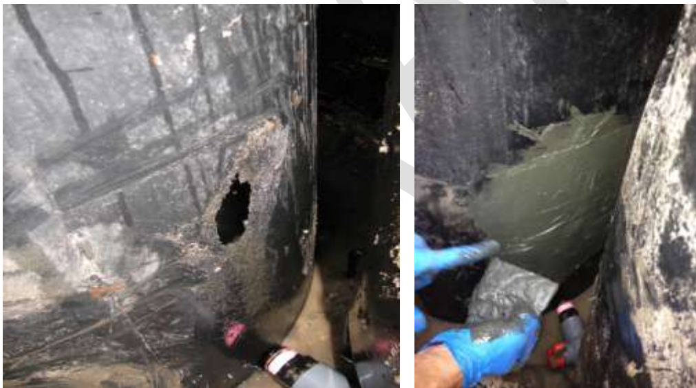
Figure 25-21. Example of animal damage to cistern and patching of hole. (NCSU BAE)
