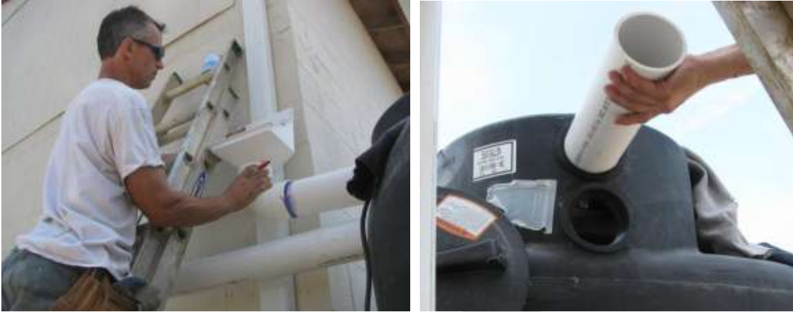
Figure 25-19. (a) Pipe leading from debris filter to the tank; (b) Rubber gasket used to create leak-free seal when pipe enters the tank. (NCSU-BAE)
