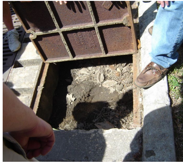
Clogged Sand Chamber
