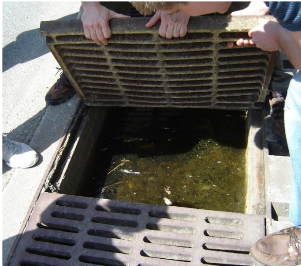
Clogged Sediment Chamber
