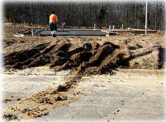
Figure 8 – Poor Construction Entrance
