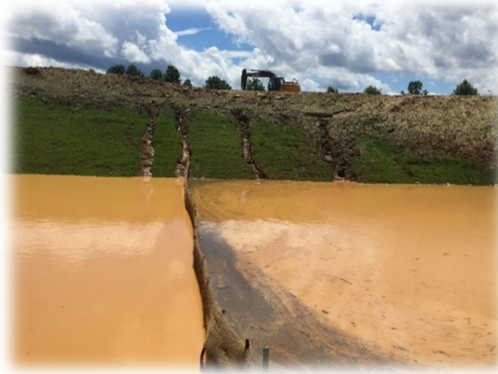
Figure 11 - Rill Erosion on Sediment Basin Slope
