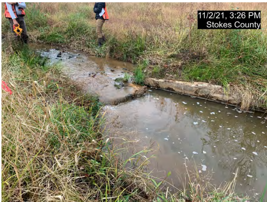
SPA-3 – BB-R3, Rock roller not functioning as intended @ STA 72+00 (MY-01)
