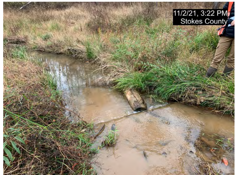
SPA-2 – BB-R3, Erosion around log vane @ STA 70+50 (MY-01)
