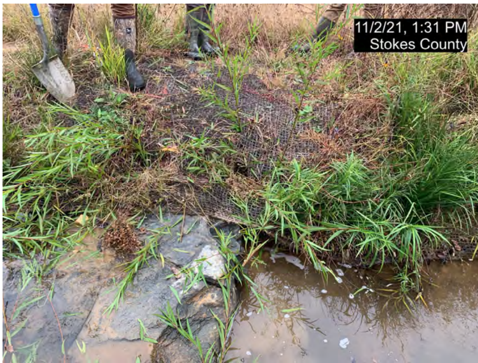
SPA-1 – BB-R1, Piping around rock structure @ STA 44+00 (MY-01)
