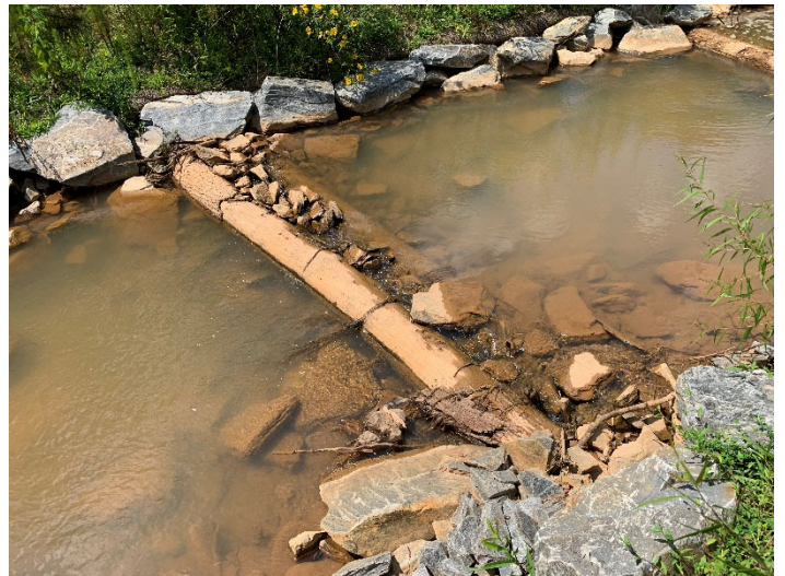
Bull Creek Reach 3: Header Dislocated from Footer at Station 164+07 – looking upstream (08/26/2021)
