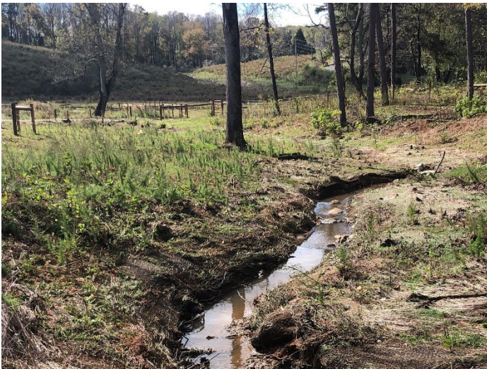
Pre-Repair – STA 405+40 – 405+65 Downstream; Riffle Scour (11/02/2020)
