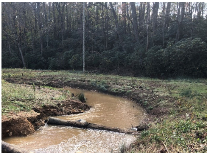
Pre-Repair – STA 106+35 Downstream; Erosion Along Right Bank Underneath Matting Possible Brush Toe Failure (11/02/2020)
