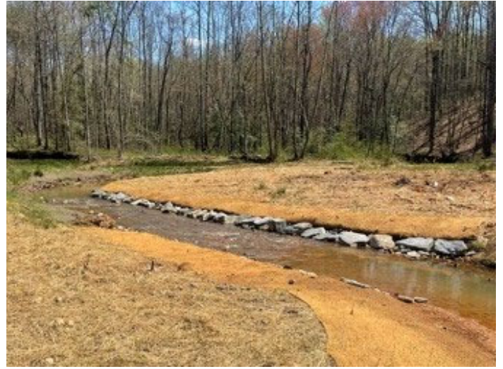
Post-Repair – STA 165+30 Downstream; Right Bank Regraded and Matted; Left Bank Seeded and Matted due to Construction Access (04/07/2021)
