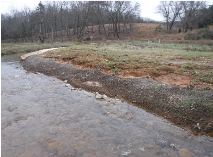
Pre-Repair – STA 152+10 Downstream; Erosion along Right Bank (12/30/2020)
