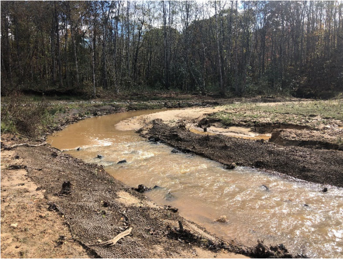
Pre-Repair – STA 165+30 Downstream; Erosion Along Right Bank (11/02/2020)
