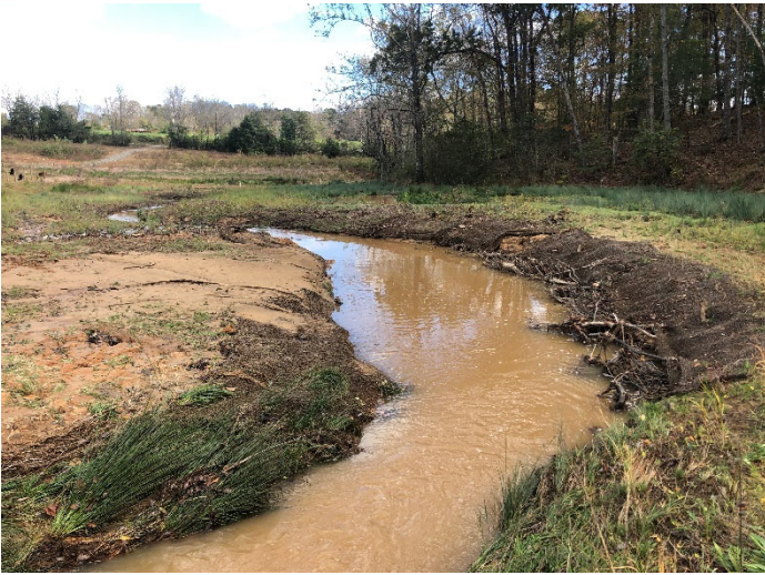
Pre-Repair – STA 112+00 Downstream; Erosion Along Right Bank Above and Within Brush Toe (11/02/2020)
