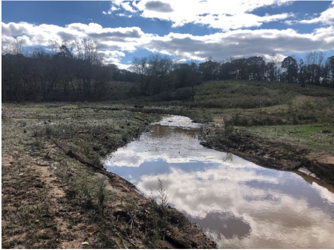
Pre-Repair – STA 150+30 Downstream; Erosion along Right and Left Banks (11/02/2020)
