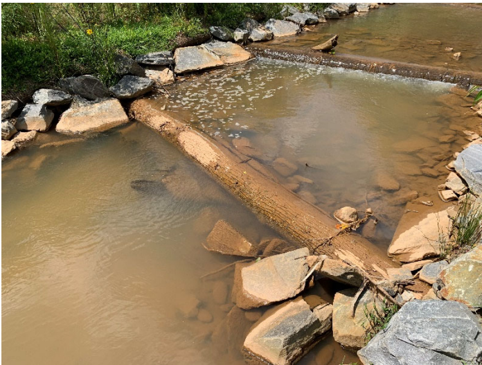
Bull Creek Reach 3: Piping at Station 164+00– looking upstream (08/26/2021)
