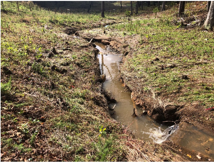
Pre-Repair – STA 404+90 – 405+30 Downstream; Riffle Scour (11/02/2020)
