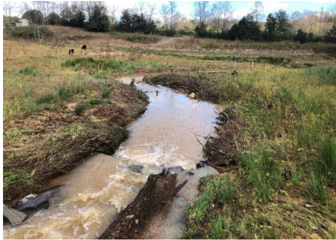
Pre-Repair – STA 113+40 – 113+80 Downstream; Riffle Scour and Erosion Along Left Bank at Riffle and Along Right Bank from Riffle Through the Brush Toe (11/02/2020)
