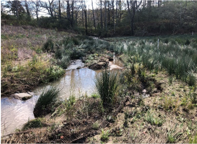
Pre-Repair – STA 212+80 Downstream; Erosion Along Right Bank (11/02/2020)
