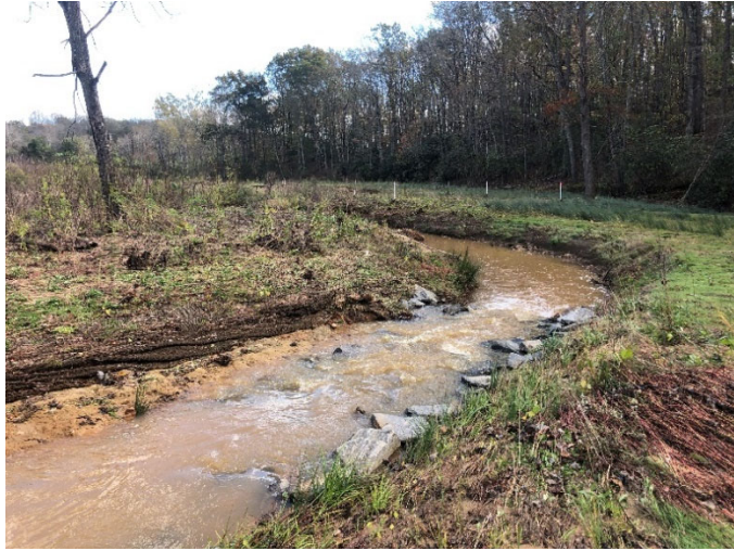
Pre-Repair – STA 107+90 Downstream; Erosion Along Right and Left Banks STA 108+20 Downstream; Erosion Along Right Bank and Brush Toe (11/02/2020)
