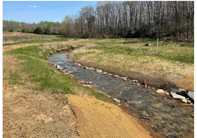
Post-Repair – STA 108+70 Downstream; Rebuilt Riffle, Reset Log Sill, and Regraded and Matted Right Bank (04/07/2021)
