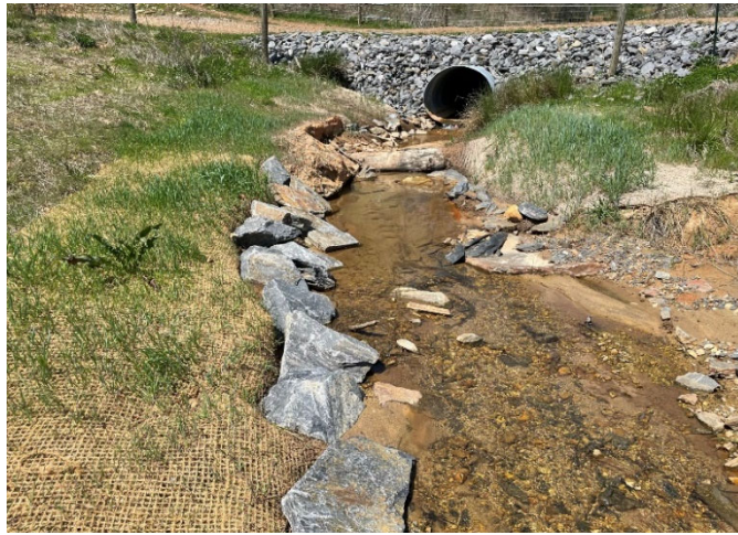
Post-Repair – STA 211+50 Upstream; Repaired Crossing Around Downstream Side of Culvert and Added Rip Rap on Downstream Face of Crossing; Right Bank Repaired and Boulder Toe Installed (04/07/2021)
