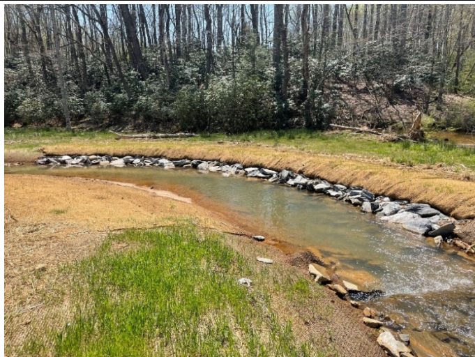
Post-Repair – STA 106+35 Downstream; Replaced Brush Toe on Right Bank with Geolift and Boulder Toe (04/07/2021)
