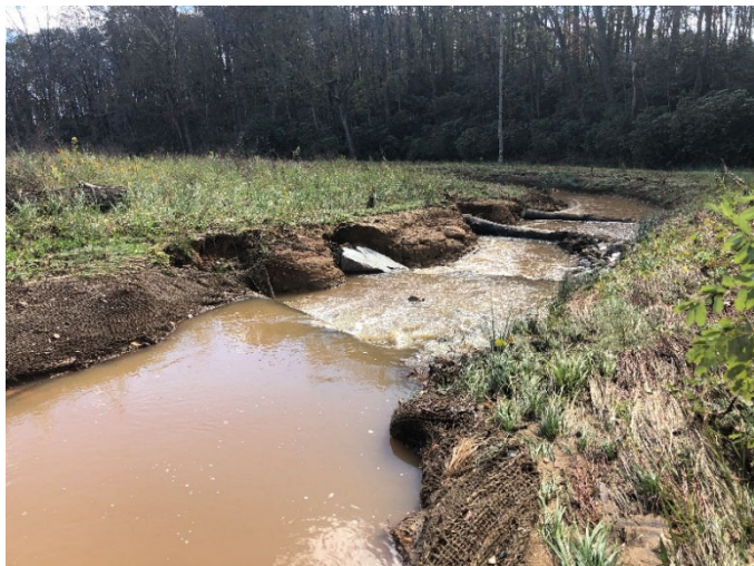
Pre-Repair – STA 105+85 Downstream; Erosion Along Left Bank at Structure Tie-ins and Loss of Riffle Material (11/02/2020)
