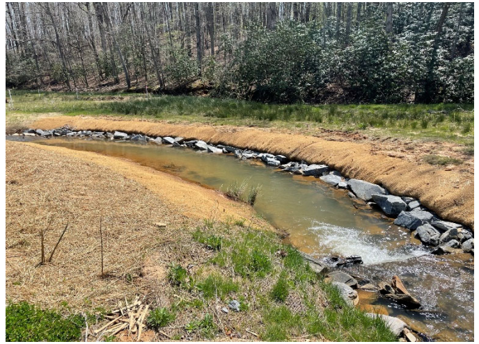
Post-Repair – STA 108+20 Downstream; Right Bank Replaced Brush Toe with Geolift and Boulder Toe (04/07/2021)
