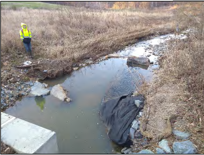
Damaged boulder sill – 12/18/20
