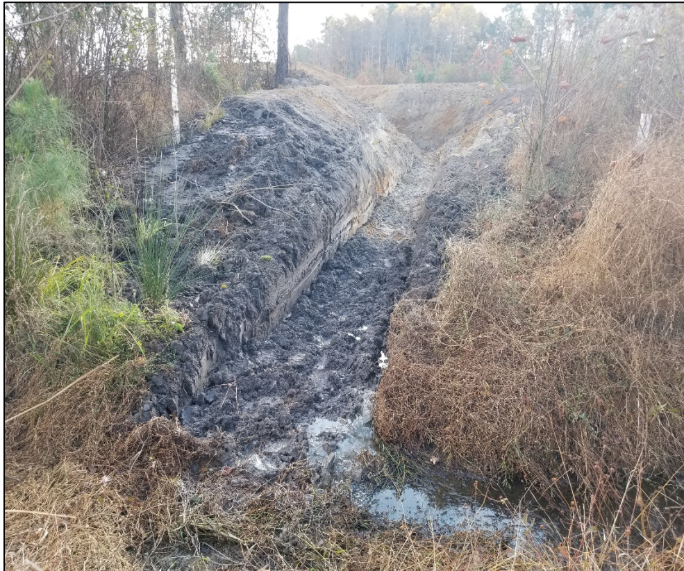
Photo 2 – View of encroachment from left bank of project stream
