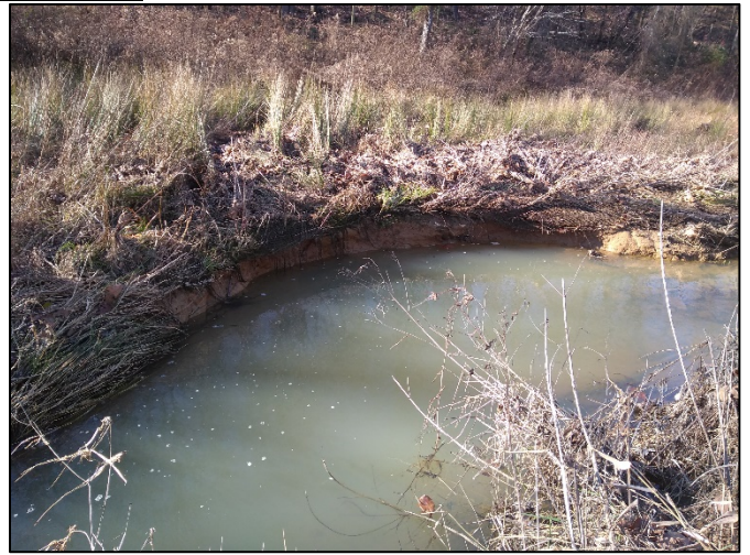
Outer bend erosion, Sta 46+25, 12/18/20
