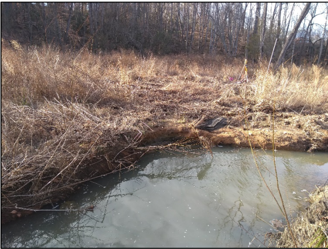
Outer bend erosion, Sta 50+75, 12/18/20
