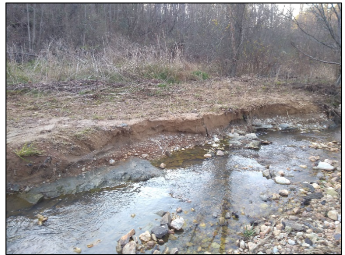
Outer bend erosion, Sta 61+00, 12/18/20
