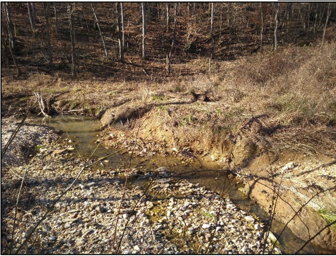
Outer bend erosion, Sta 39+50, 12/18/20
