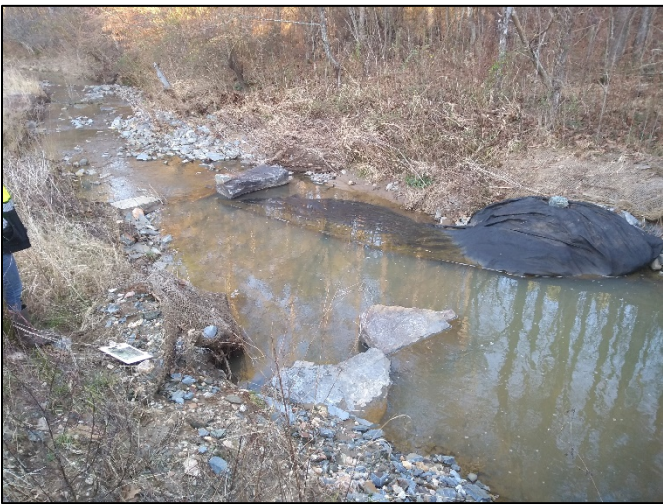
Damaged boulder sill, Sta 55+60, 12/18/20
