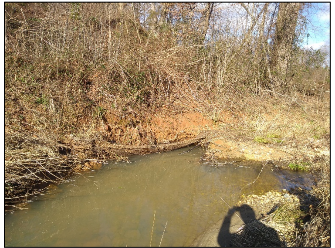
Outer bend erosion, Sta 54+25, 12/18/20
