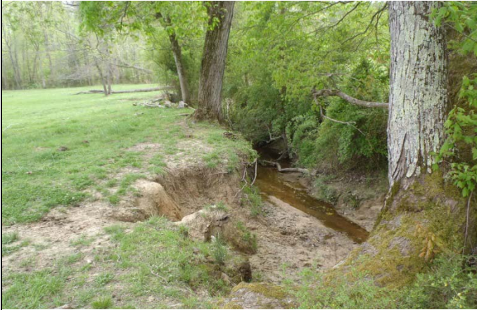
View looking at incised and eroding channel along Reach R1 (4/16/2013)
