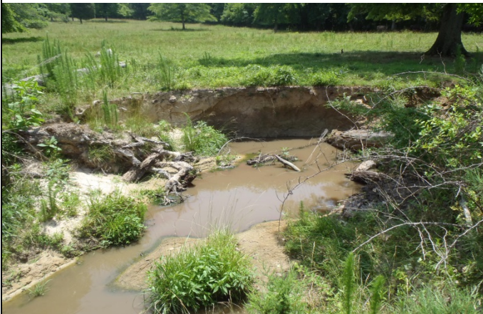
View looking downstream at channel incision with vertical eroding bank along Reach R1 (6/19/2014)
