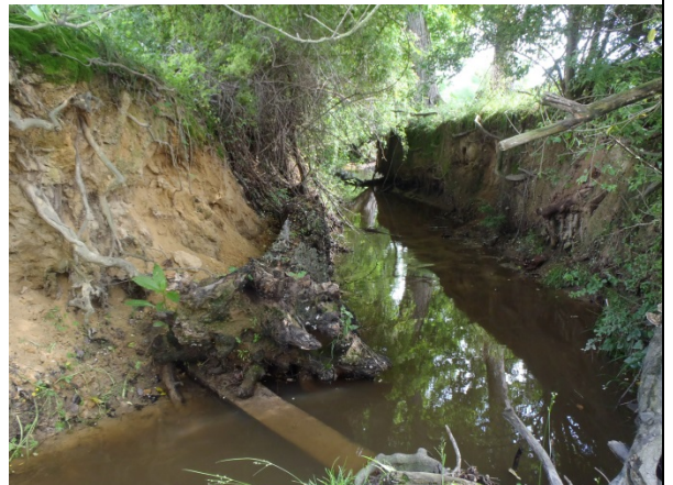
View looking upstream at cross section of Reach 1 with channel incision and eroding banks (4/22/13)
