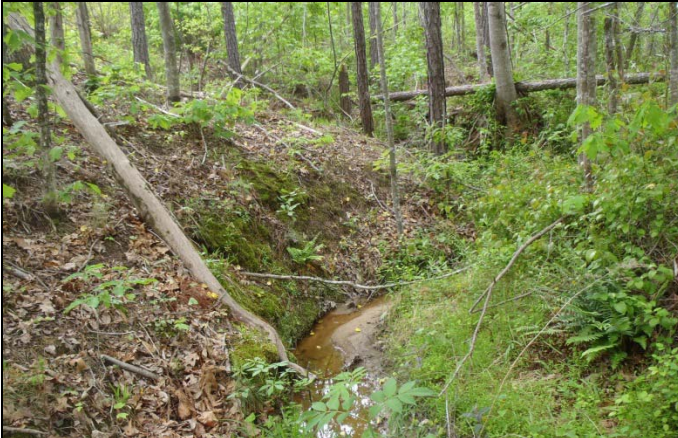
View looking upstream along Reach R7. This area is targeted for supplemental buffer planting only. (5/8/13)
