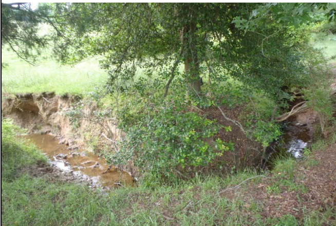
View looking at incised channel, eroding outside bend, and minimal buffer along lower Reach R2 (5/22/13)
