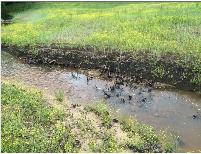
Repaired Stream Area (before), May 2016, Station 42+50
