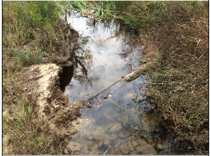
Stream Problem Area (downstream), Oct. 2016, Station 40+60
